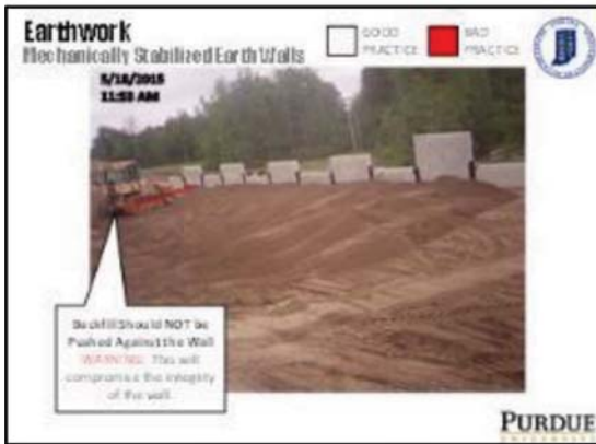
(e) Poor practice for MSE earthwork
