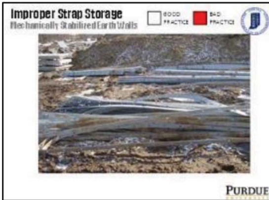
(c) Bad practice for reinforcement straps
