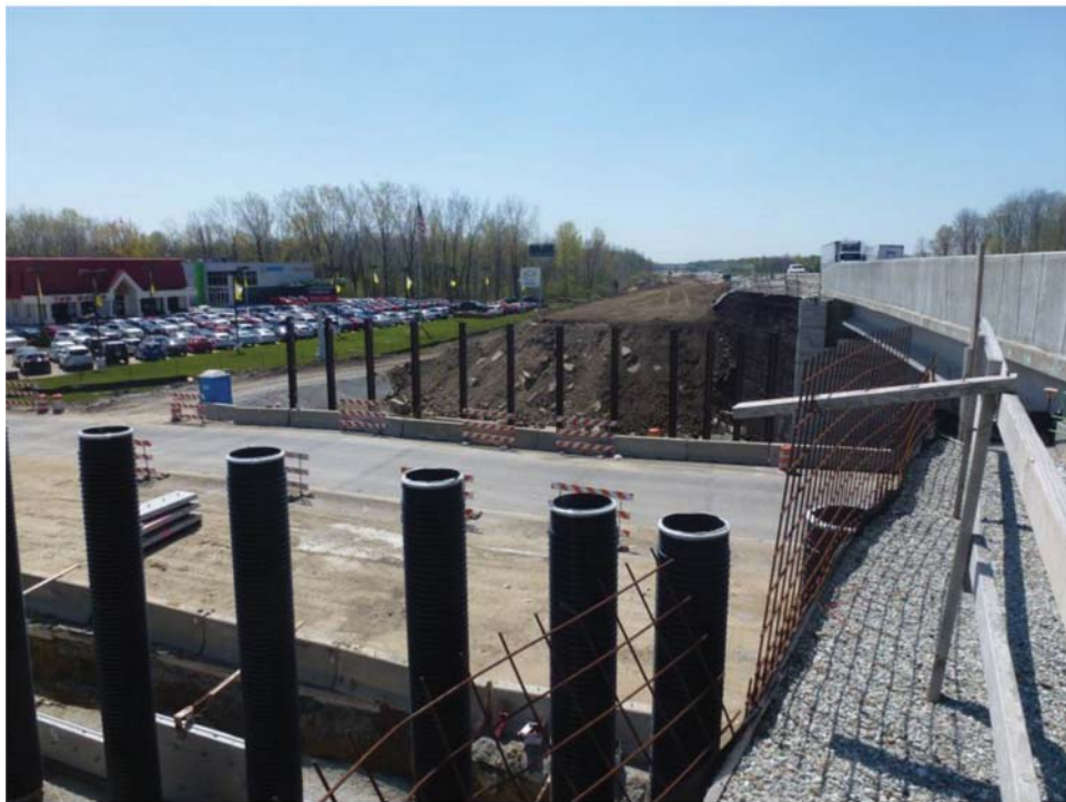
(b) View of uncovered H-piles and covered H-piles from time-lapse camera location
