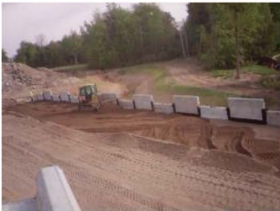
(c) Soil near panels is pushed along the length of the panels
