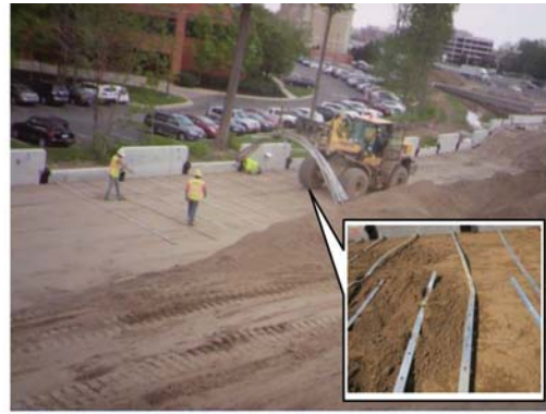
(b) Driving over straps causes damage
