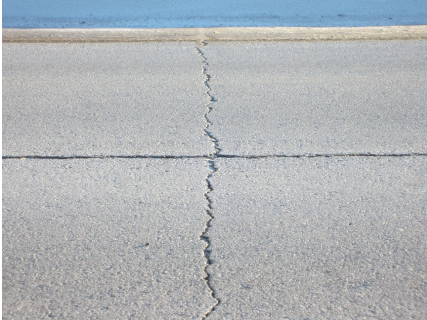
TH 210-typical crack configuration
