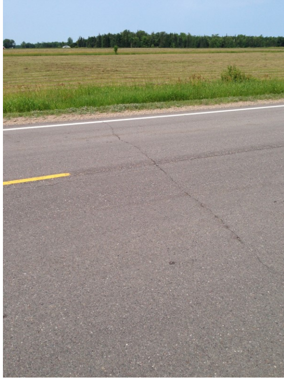
CSAH 10 good performer: typical crack configuration
