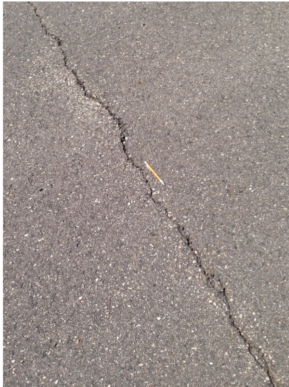
TH 220-typical crack profile
