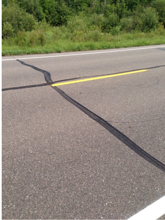
TH 6-typical crack configuration
