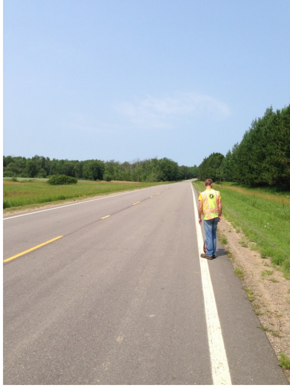
CSAH 10 poor performer-overview
