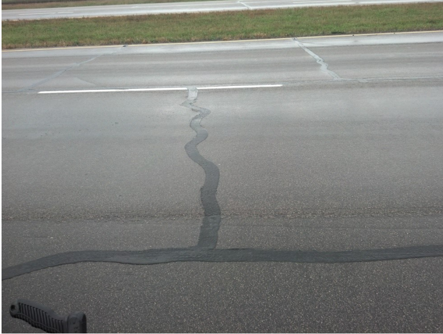
TH 10 poor performer-typical crack configuration
