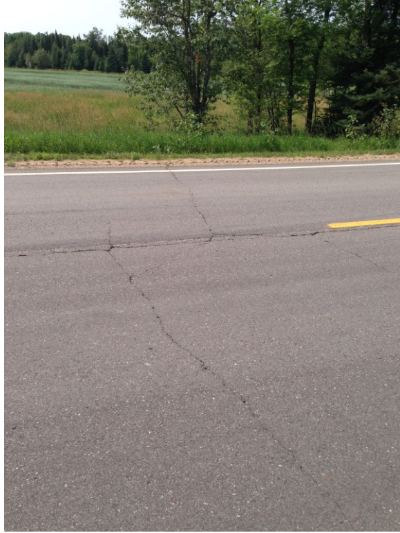
CSAH 10 poor performer: typical crack configuration
