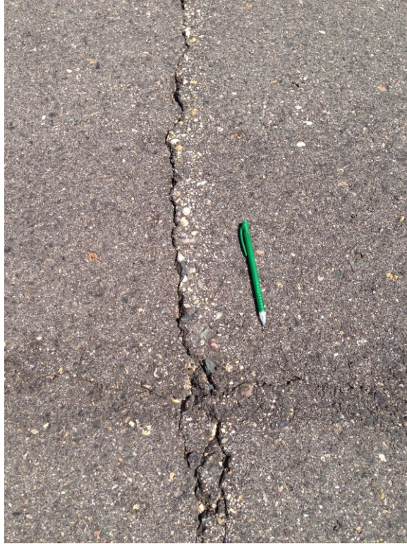
TH 10-typical crack profile
