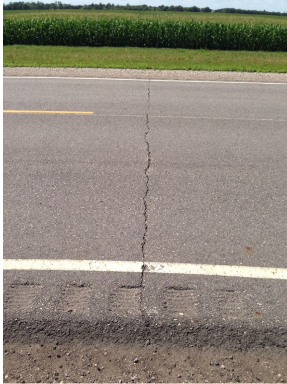
TH 220-typical crack configuration
