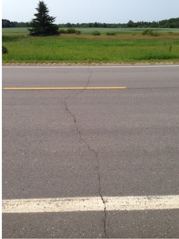
CSAH 10 poor performer-typical crack profile
