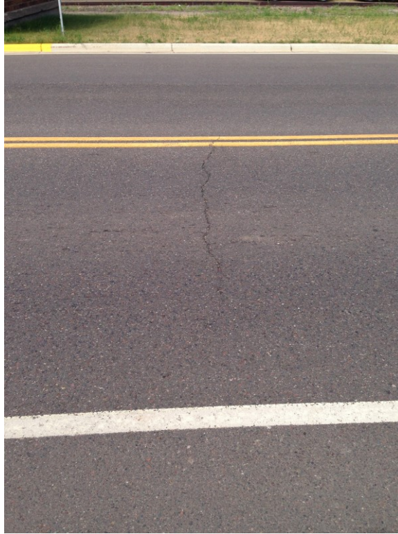
CSAH 30-typical crack profile
