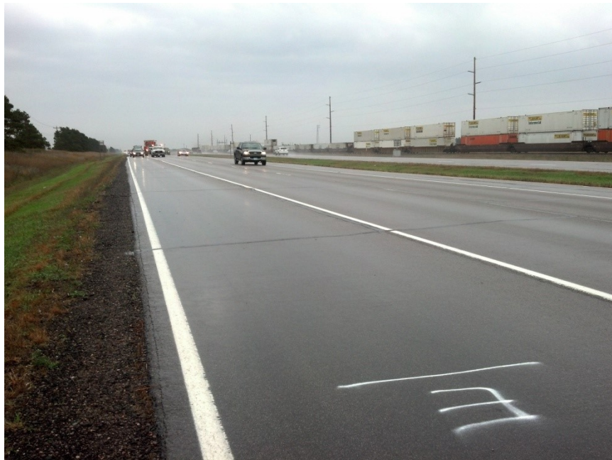
TH 10 poor performer-overview
