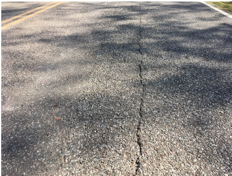
Figure 9. Longitudinal cracking in the wheel path of an existing HMA pavement.
