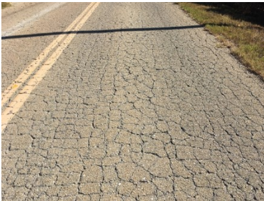
Figure 8. High-severity fatigue cracking in HMA that is not suitable for BCOA designs unless milling will expose HMA in fair to good condition.
