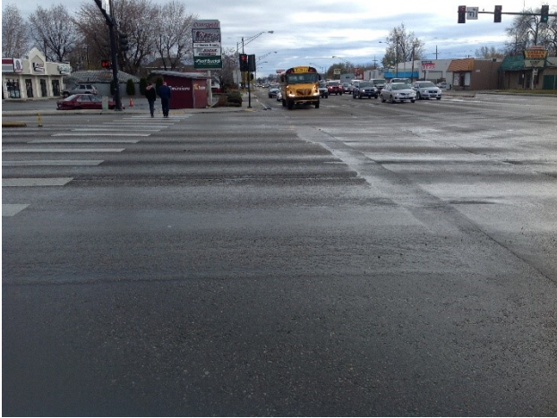
Figure 13. Rutting in HMA evidenced by standing water in the wheel paths.
