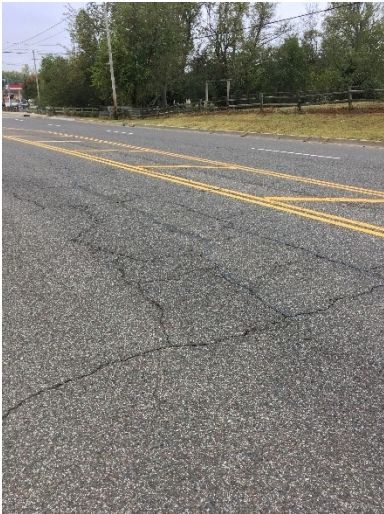
Figure 7. Moderate-severity fatigue cracking in HMA that is not an issue for BCOA designs.
