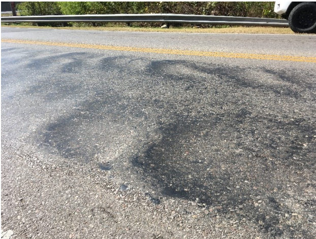
Figure 14. Shoving in HMA pavement at an intersection approach.
