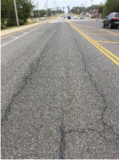
Figure 6. Low-severity fatigue cracking in HMA that is not an issue for BCOA designs.
