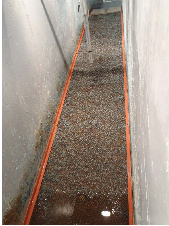
Figure 4.84. View looking upstream after six hours of run time. Almost all of the FRM has been washed away and the depression near the shoulder has gotten deeper.
