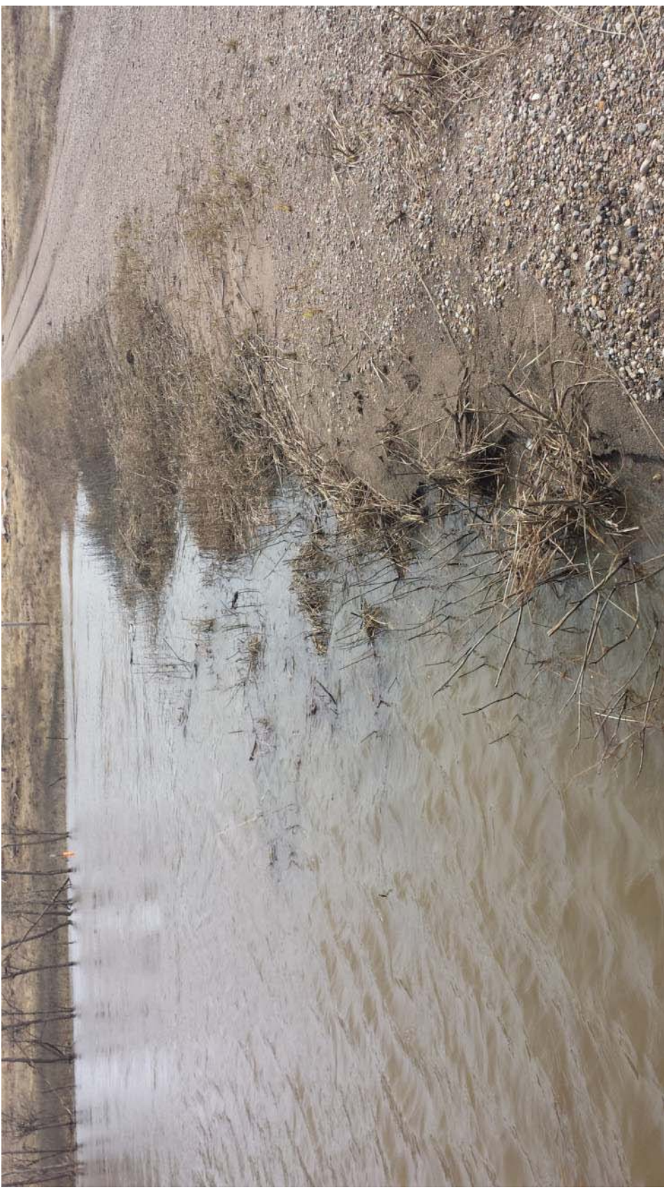
Location 4 looking east at minor erosion and deposition on the downstream shoulder, post-flooding condition
