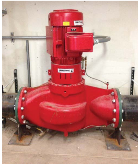
Figure 3.4. Pump #1 on the model floor.
