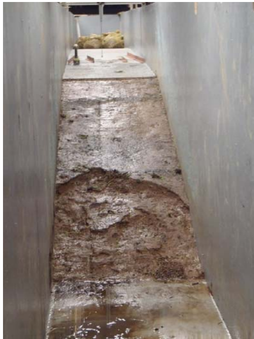
Figure 4.57. Looking upstream from run-out area. Stabilization material removed showing the extent of the erosion starting at the toe of the slope and working up towards the shoulder.
