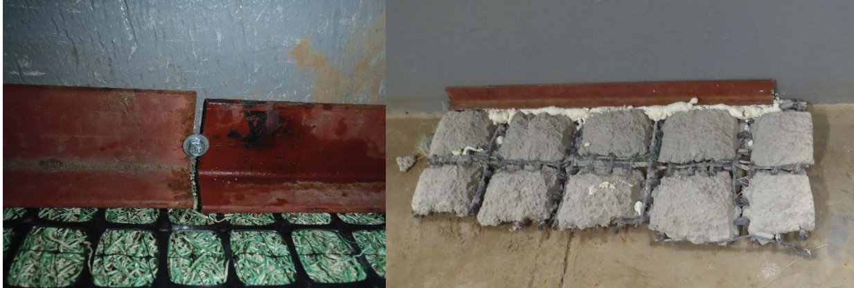
Figure 3.18. Angle iron fastened to flume wall (left). Flexible concrete geogrid mat installation example with backer rod and spray foam insulation used to fill the void between the Flexamat ® and angle iron resting on top of concrete (right).
