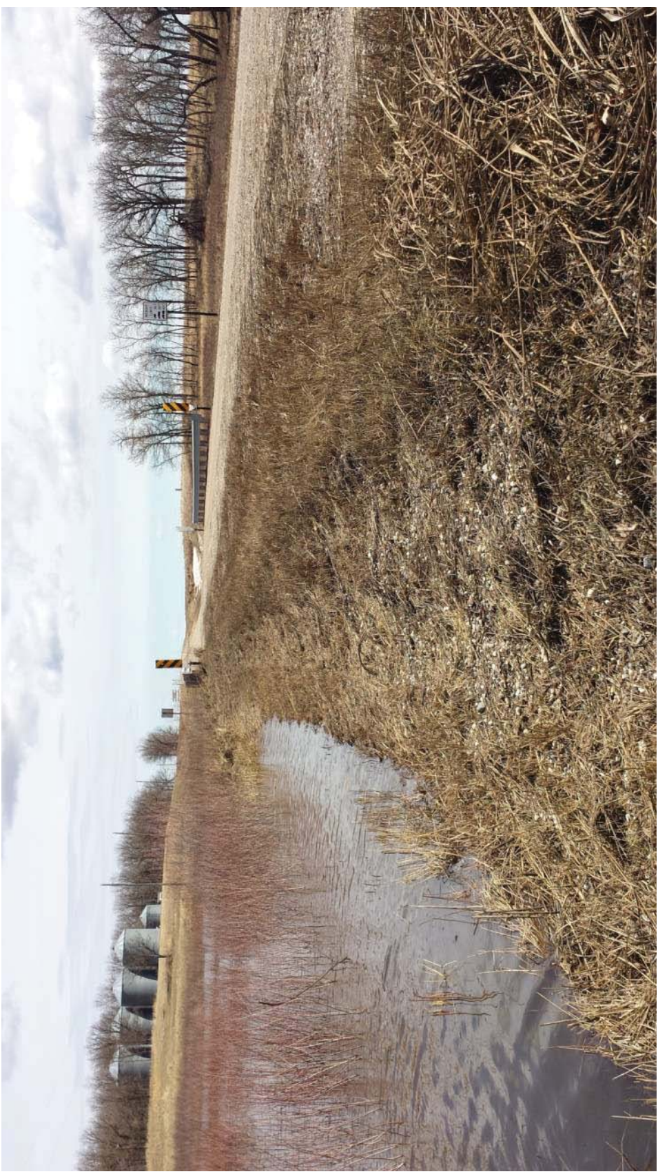
Location 5 Looking east at the upstream shoulder, post-flooding condition
