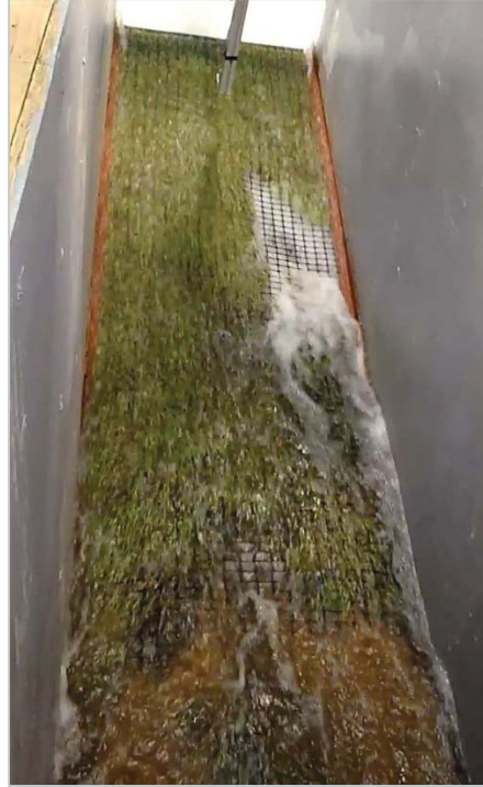
Figure 4.65. During final 4-5.5 hour run, catastrophic erosion took place. Most of the lower slope began eroding under the sod, which had come loose but was held from being washed away by the geogrid and staples.
