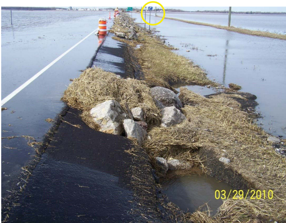
Figure 1.5. Same location, eight days later. Temporary stone fill dumped in some scour holes. Photo by JT Anderson, MnDOT.
