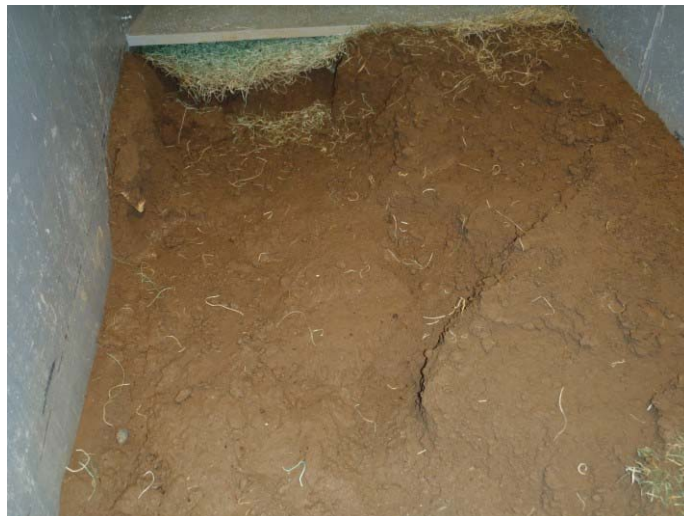
Figure 4.23. Slope with the shoulder at the top of the photo after ECB was removed post-testing. Note the undermining of shoulder and extensive erosion not seen with ECB still in place on previous photos.
