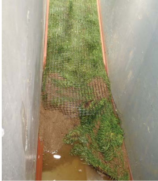
Figure 4.56. Looking upstream at toe of slope. Erosion beginning at toe of slope, undermining sod and washing some pieces away. Erosion working up the slope from run-out area.
