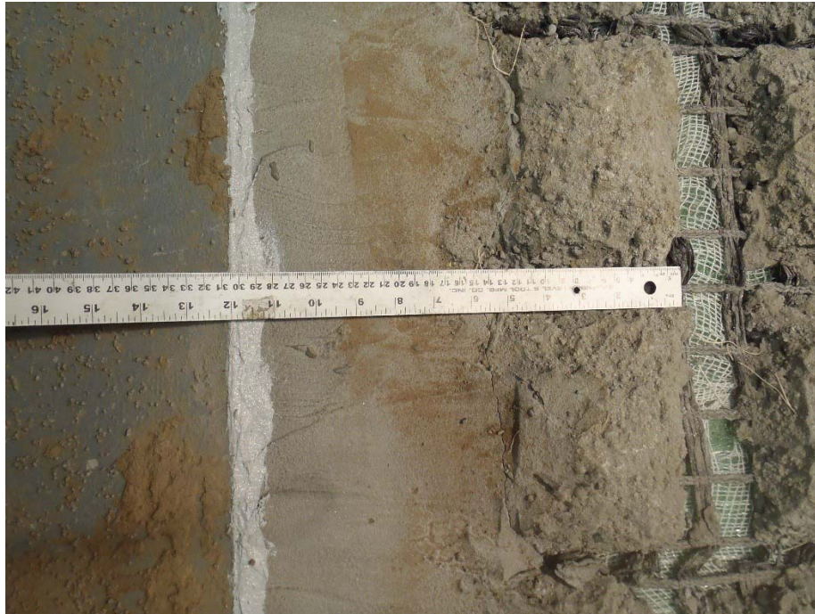
Figure 3.17. Flexamat® “paved” into the shoulder with Portland cement grout to transition onto the slope. Seam of paving and shoulder sealed with a polyurethane single component sealant (white). Flow is left to right in this image.
