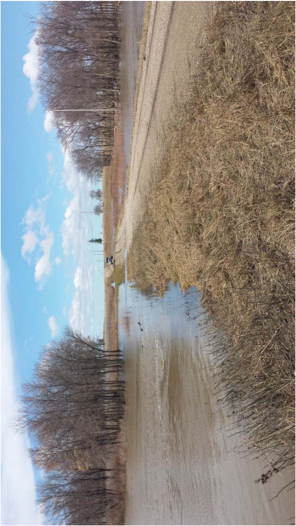
Location 4 Looking west at the upstream shoulder, post-flooding condition
