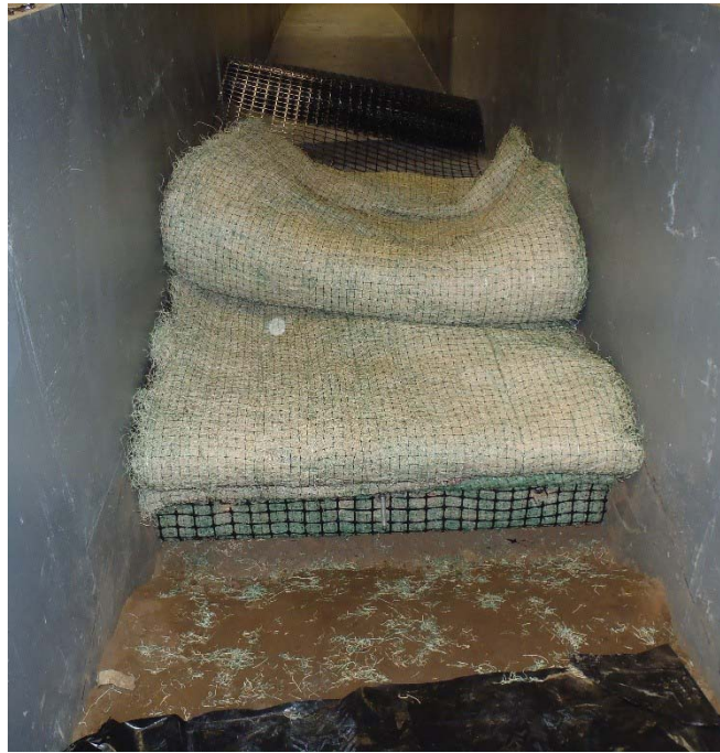
Figure 3.15. View looking upslope. Armored sod material wrapped around a piece of lumber and bolted to framing under the shoulder. Once backfilled with soil, the armored sod material on the shoulder would be flipped down to cover the slope.
