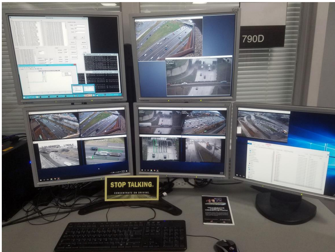
Figure 2.5 QWARN Monitoring Station at the MTO
