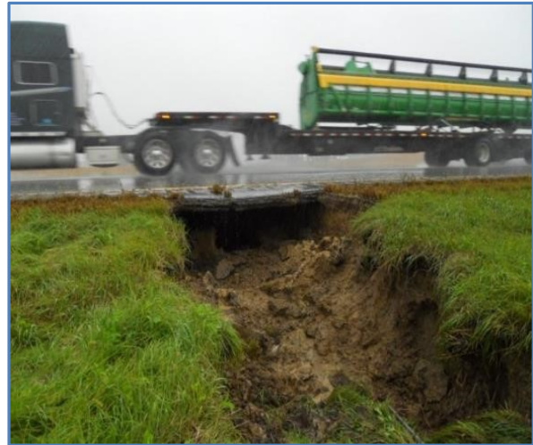
Figure 1.1 – Unseen Culvert Damage
