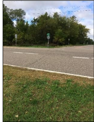
Figure 4 – A crack was observed in the road above Culvert ID 206853. This crack correlates with the culvert alignment.
