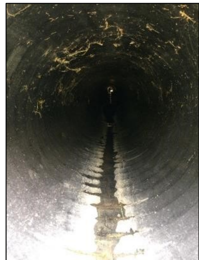
Figure 3 – Visual Inspection of Culvert ID 410672 indicates no major deformations impacting the culvert cross section.
