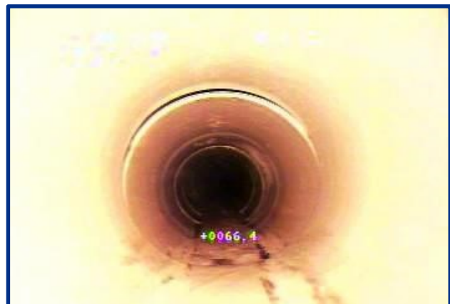
Figure 5.5 – CCTV Image with Too Much Light
