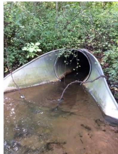
Figure 7 – Culvert ID 651309 had a severely corroded invert. The inspection camera could not travel through the culvert.
