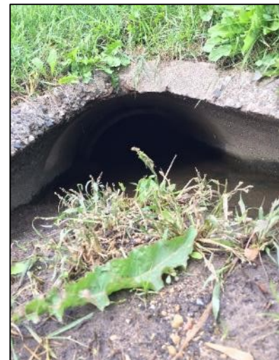
Figure 5 –Culvert ID 206853 was full of sediment. The CCTV camera could not inspect this culvert.
