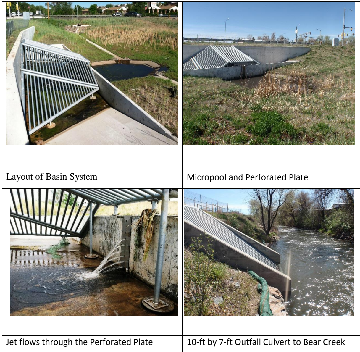
Figure 2.9 As Built EDB 502L Located at S Knox Court and SH 285.
