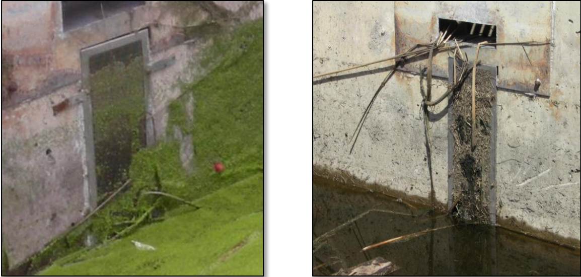
Figure 22. Typical frequent clogging issues associated with well screens (Grant Ranch Research Extended Detention Basin, Denver, CO 2009).
