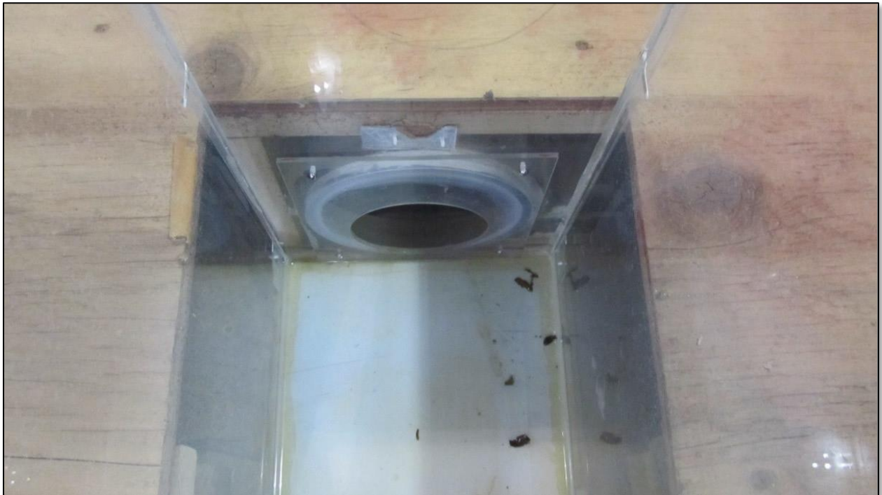
Figure 40. 100-year restrictor plate covering the final discharge pipe inside the outlet structure.
