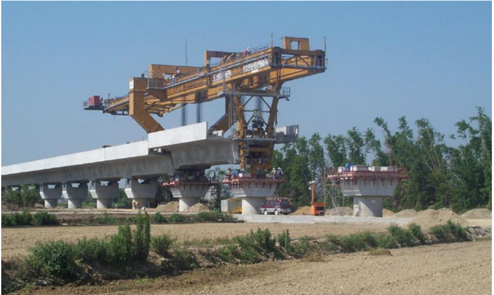
Figure 3-13: Example of Overhead Gantry
