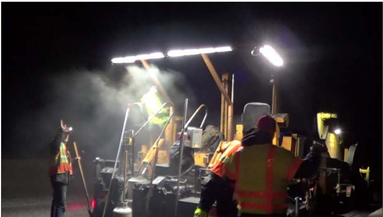
Figure 7.19: Two Workers Indicating Alarm was Heard, Case Study Project #3
