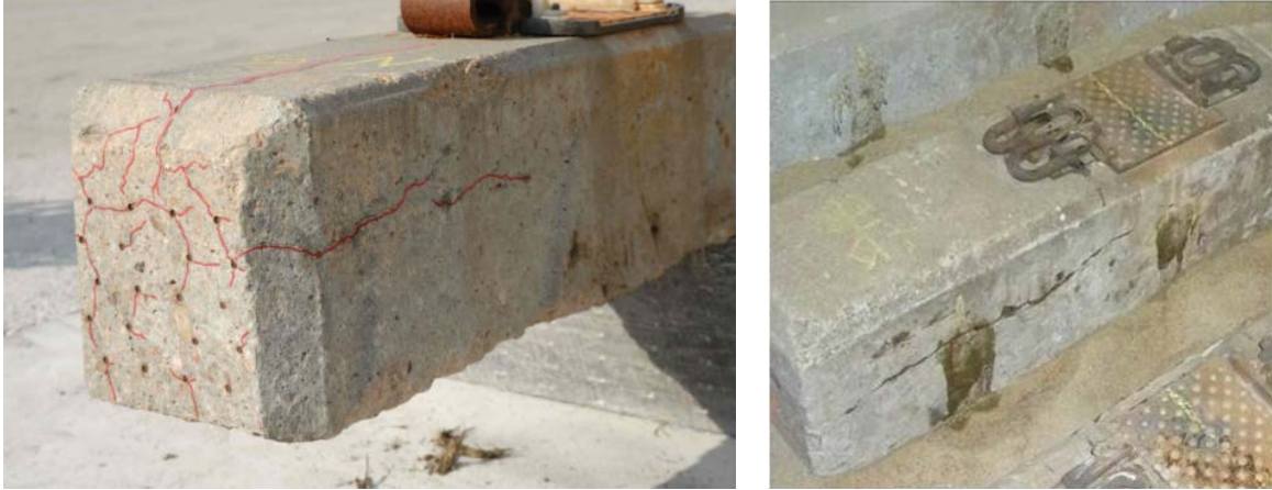
Figure 1. Examples of concrete crosstie bursting (left, 3) and splitting failures (right, 4).
