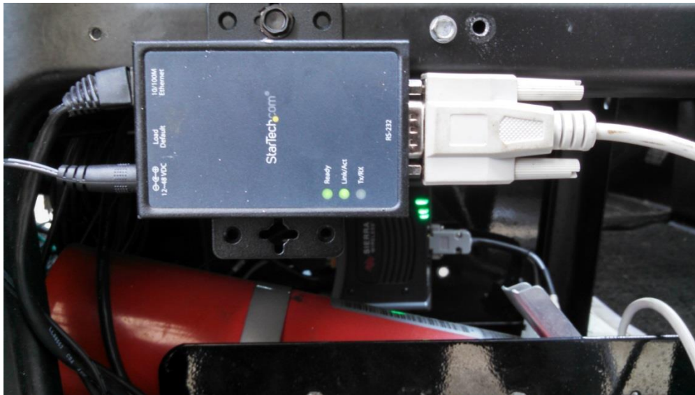
Figure A.19: Installed Ethernet to RS-232 switch.
