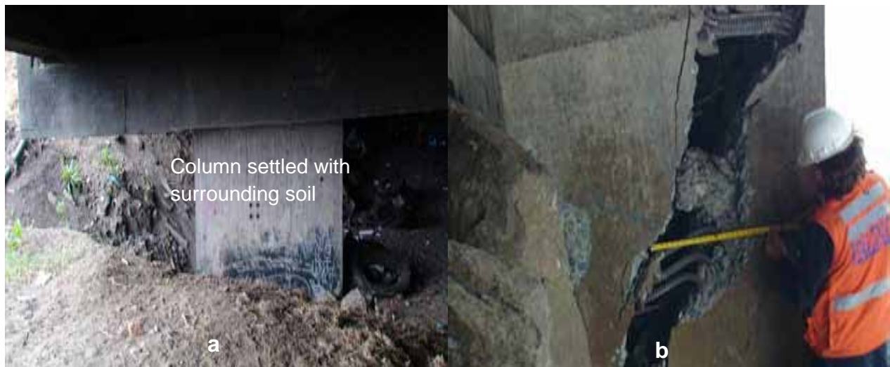
Figure 3.8. (a) Column settlement under approach and (b) back face of failure plane at northern end of Juan Pablo II Bridge (Yen et al. 2011).
