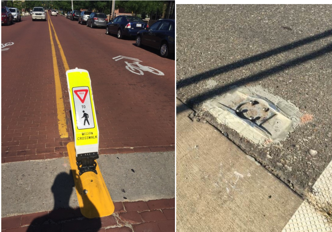
Figure 7.2. Figure 7.2a (above left) shows an R1-6 sign installed on a removable curb base that was damaged during the study. Figure 7.2b (above right) shows a sheared base of a flush mounted sign.
