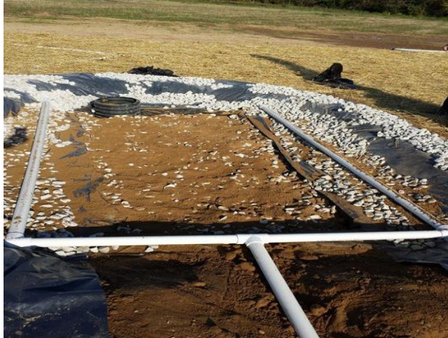
Figure 57. Sediment on 10-year-old infiltration trench.
