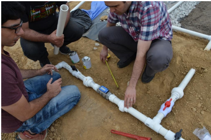
Figure 49. Flowmeter installed in the pipeline.
