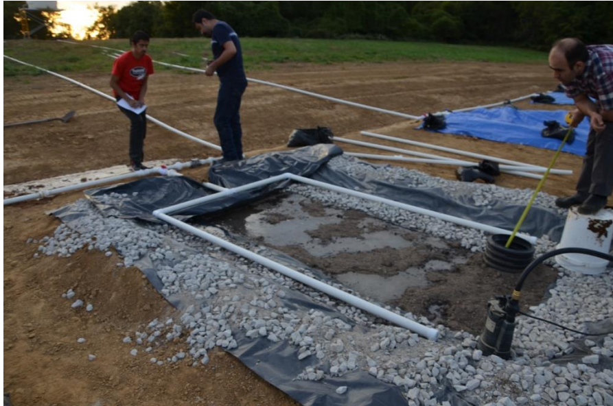
Figure 48. Piping system and bioswale during a control test.
