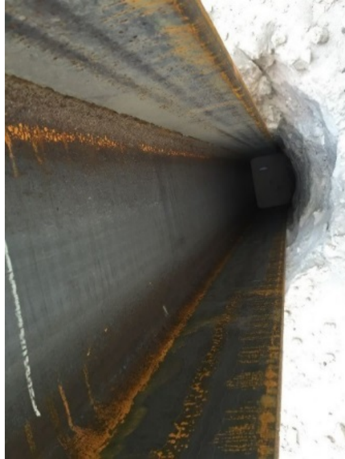
Figure 3.5 Soil gap between H-pile flanges
