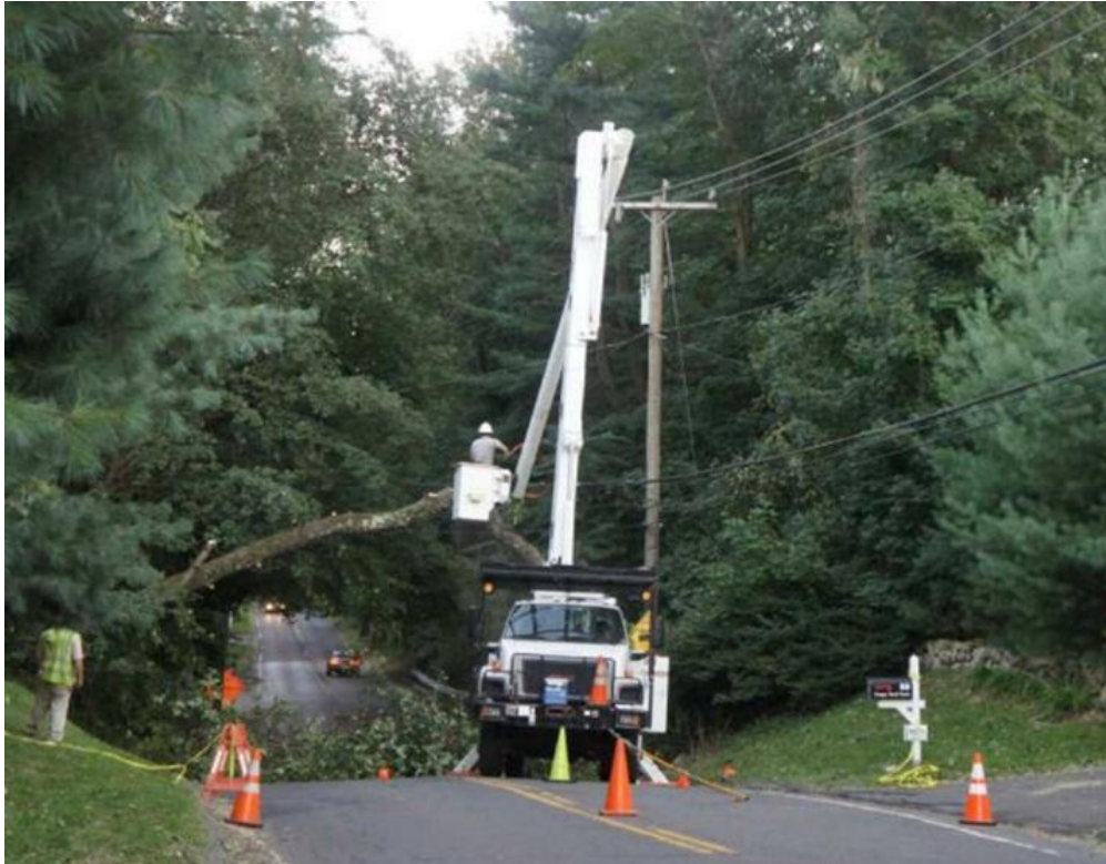
Figure 6.5 Clear Zone Reclamation after Tropical Storm Irene (2011)
