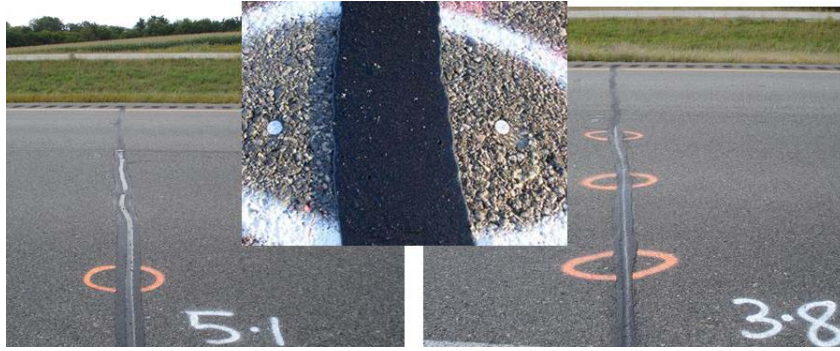
Figure 3. Crack Displacement Pins: Single-Point to Measure Only Right Wheel Path (left) and Three-Point to Measure Both Wheel Path and Middle of the Lane (right)
