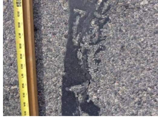
(b) Overband failure
