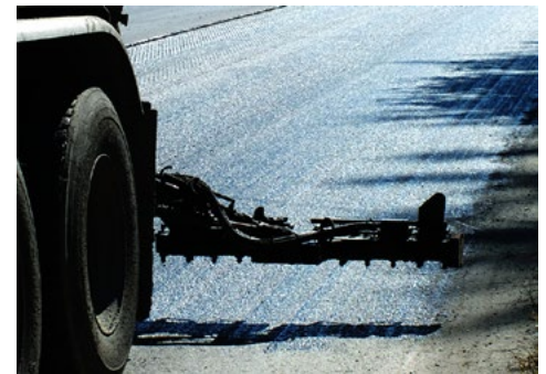
An even layer of tack coat is essential for ensuring good bonding between layers of asphalt.
