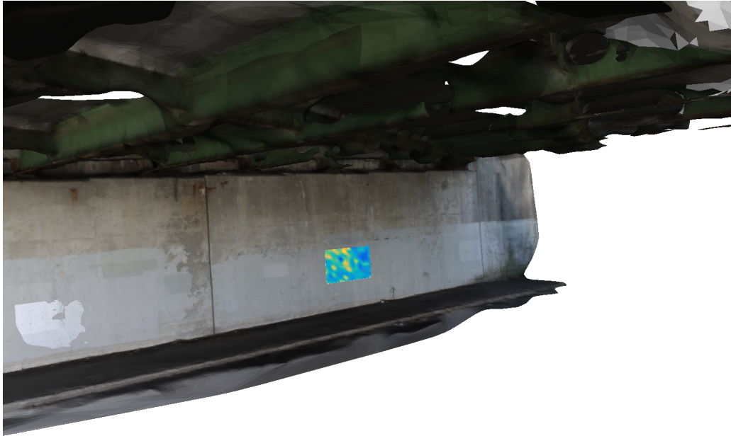
Fig. 106. Integrated 3D radar image with mechanical strength of concrete, Lincoln St. Bridge
