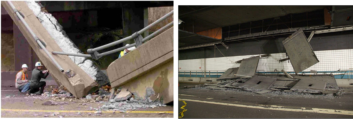
Fig. 1. Bridge and tunnel failures: (left) I-70 Lake View Drive Bridge (Pittsburgh, PA) and (right) I-93 Tunnel (Boston, MA)
