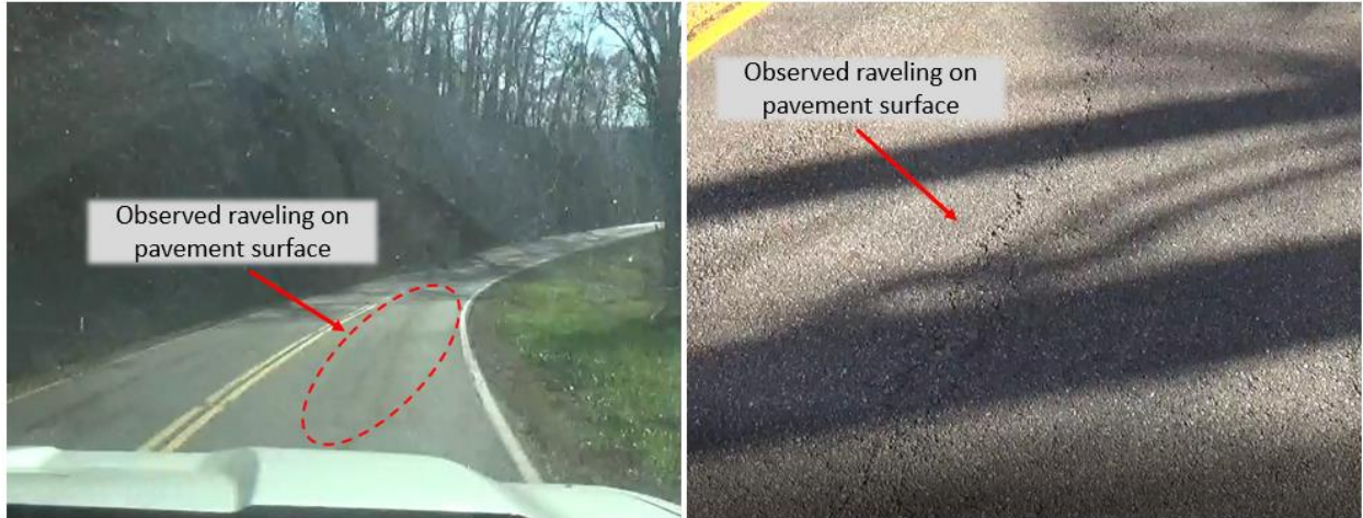
Figure 7. Raveling on Canopy Covered Pavement Sections.
