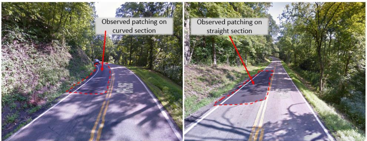
Figure 8. Patched Pavement Sections Under Canopy Cover.
