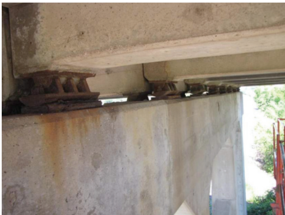
Corroded Steel Rockers Limiting the Ability of the Rockers to Rotate and Prevent the Girders from Rotating at the Supports as Designed
