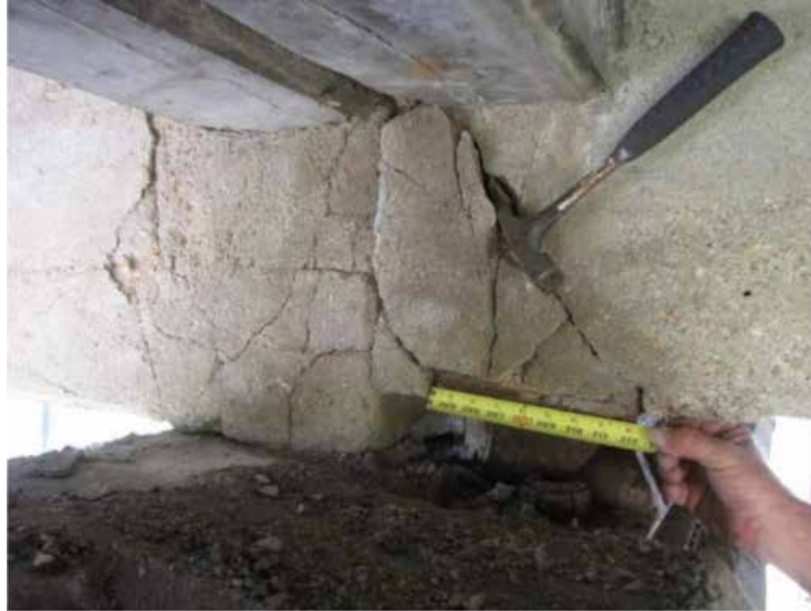
Figure 2.2: Crack Width at Girder C, Left Side, Pier 1 of Bridge No. 54-104-317.27
