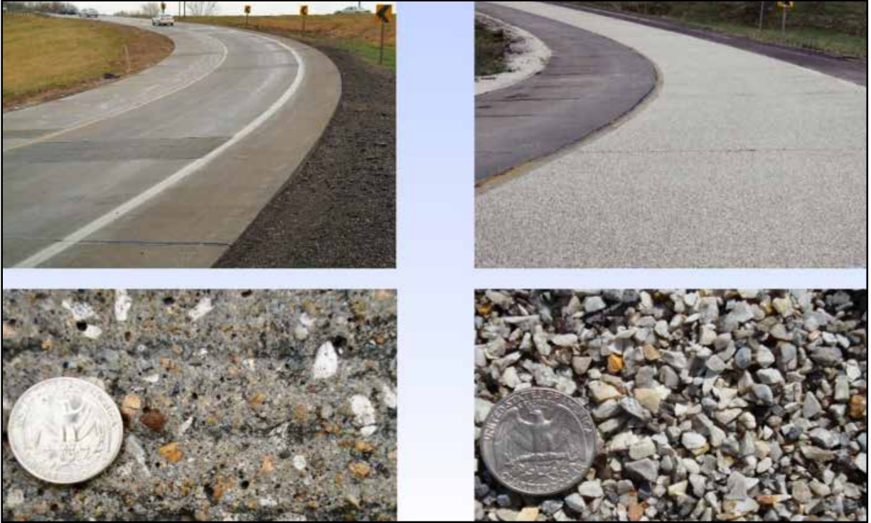
Figure 2.18: Before and After HFST on I-35/I-635 Ramp in Kansas City (Concrete Pavement)
