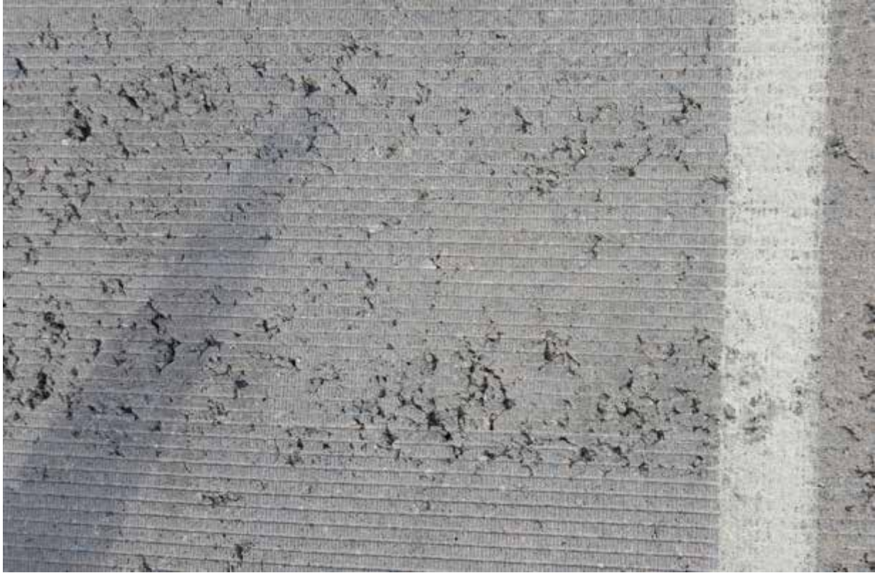
Figure 4.24: Surface Voids in LC-HPC-5 Bridge Deck
