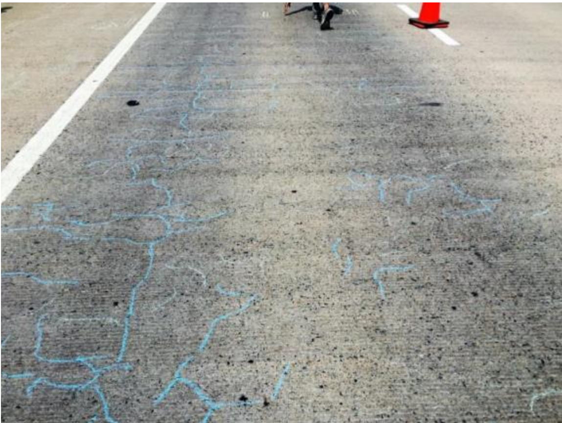
Figure 4.51: Short Map Cracks and Discolored Surface on South Lane
