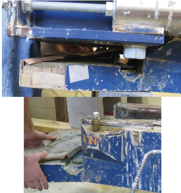
Figure C.2: Separation of copper flashing.
