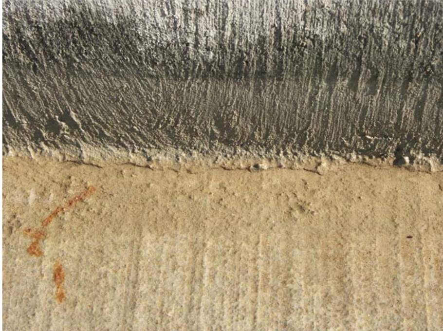
Figure 7.26: Cracking between bridge deck and sidewalk concrete.
