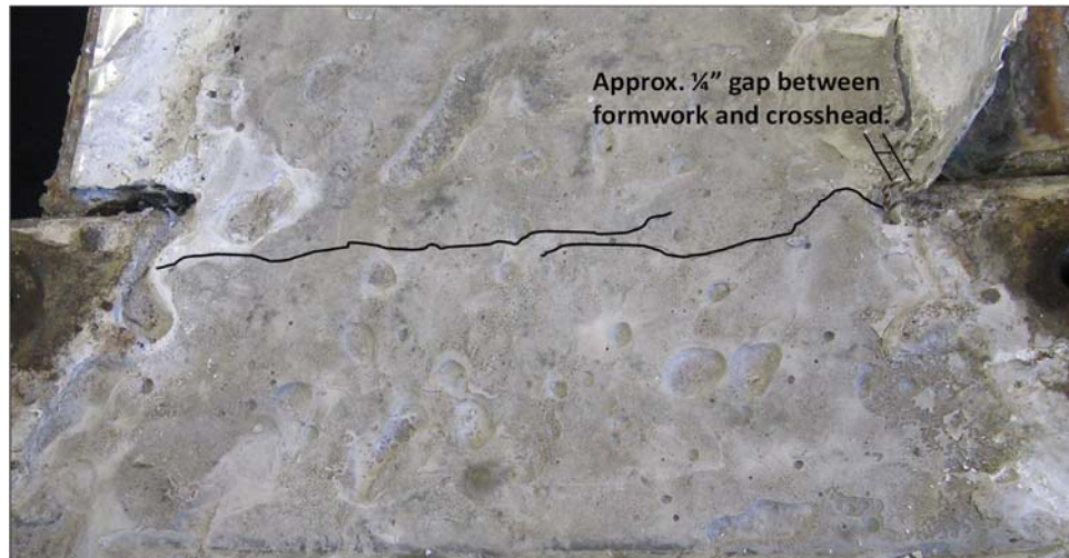
Figure C.1: Stress concentrations from formwork fatigue.
