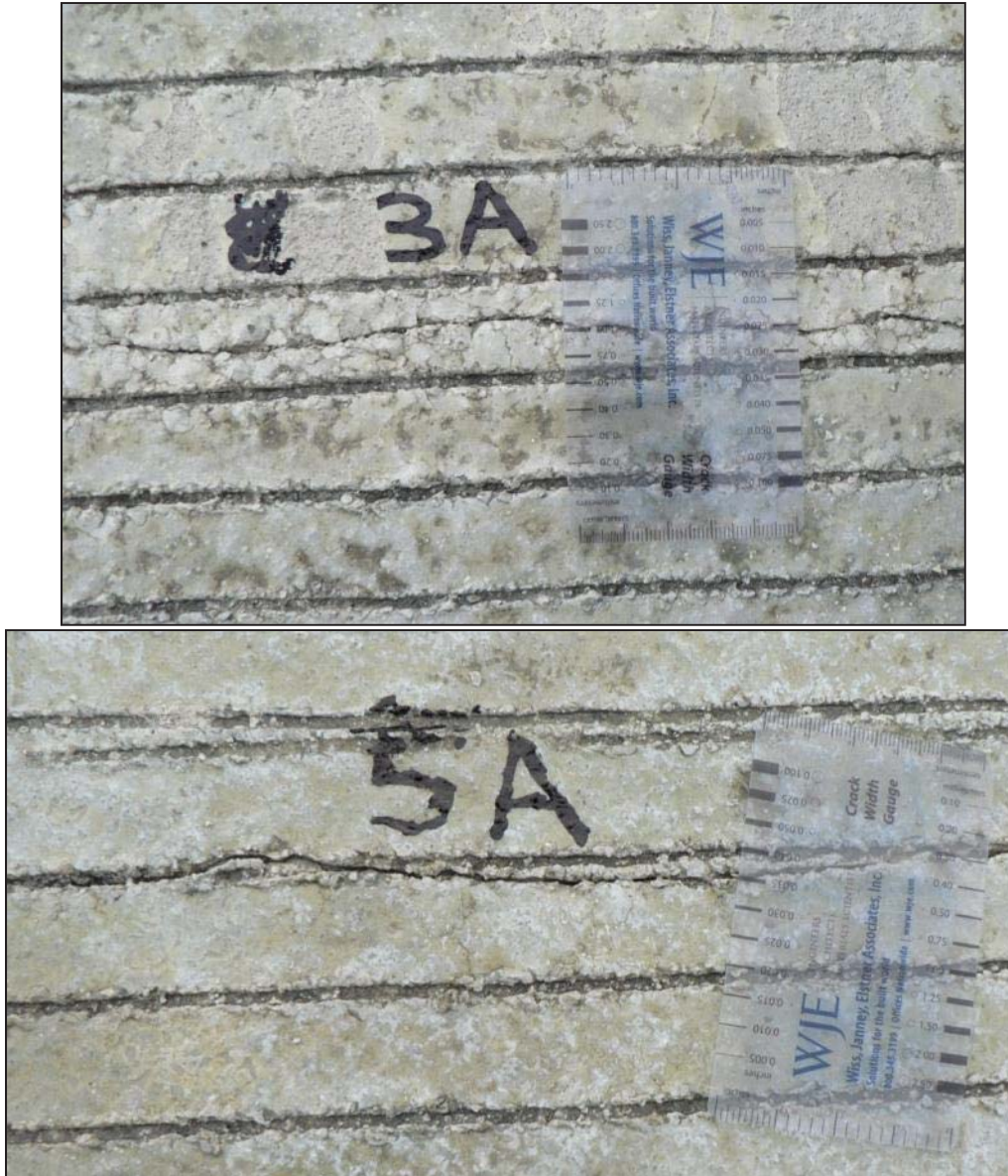
Figure 7.7: Crack-like lines on San Antonio bridge deck.
