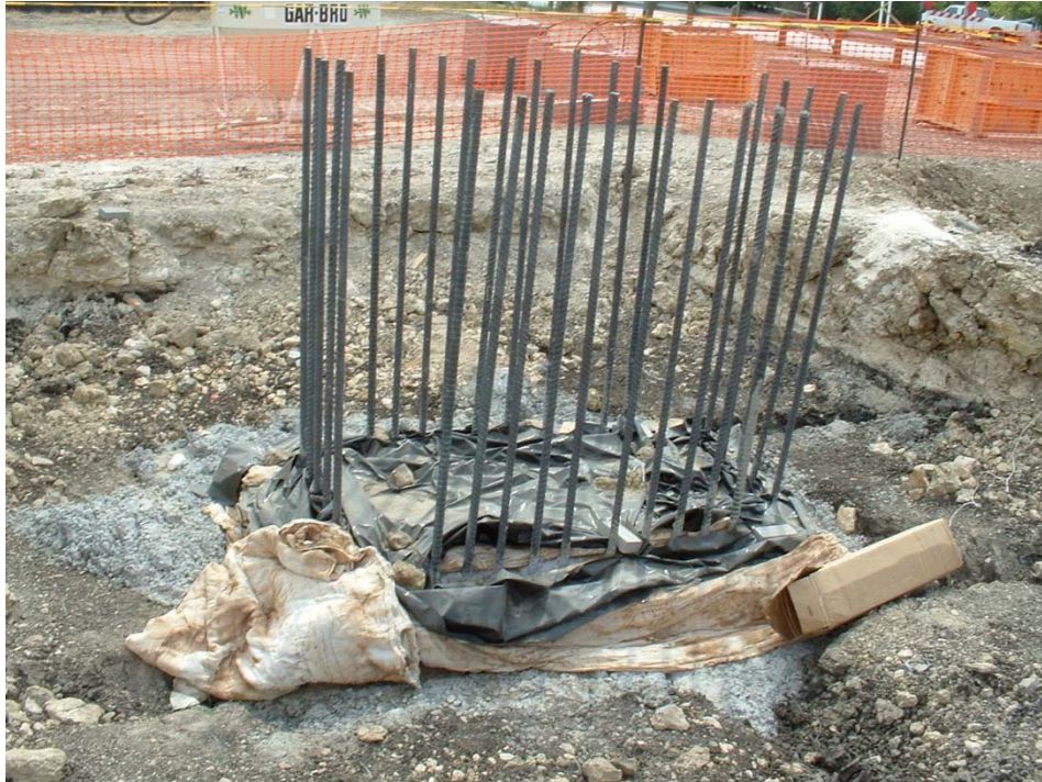
Figure 56 - Example of a footing that would use the “soil on the sides” option
