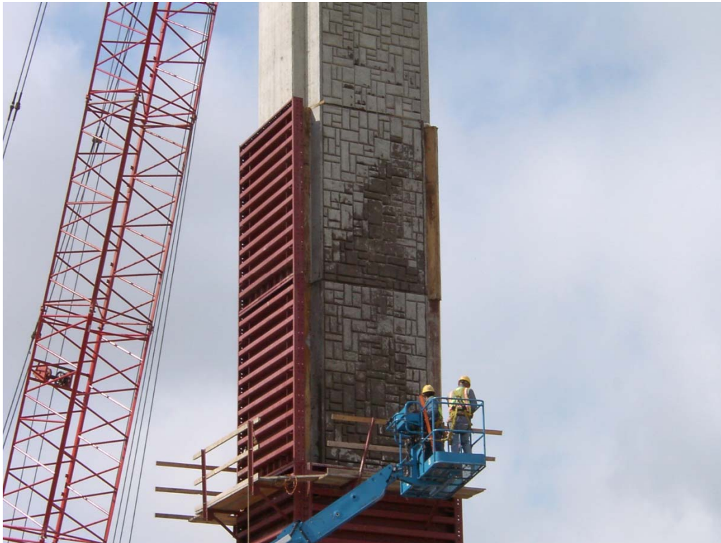
Figure 6 - Rectangular column during form removal and the beginning of construction stage two
