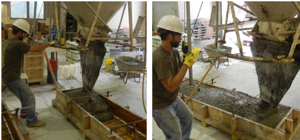
Figure 3-10: Images showing placement from one end of a slab to the other
