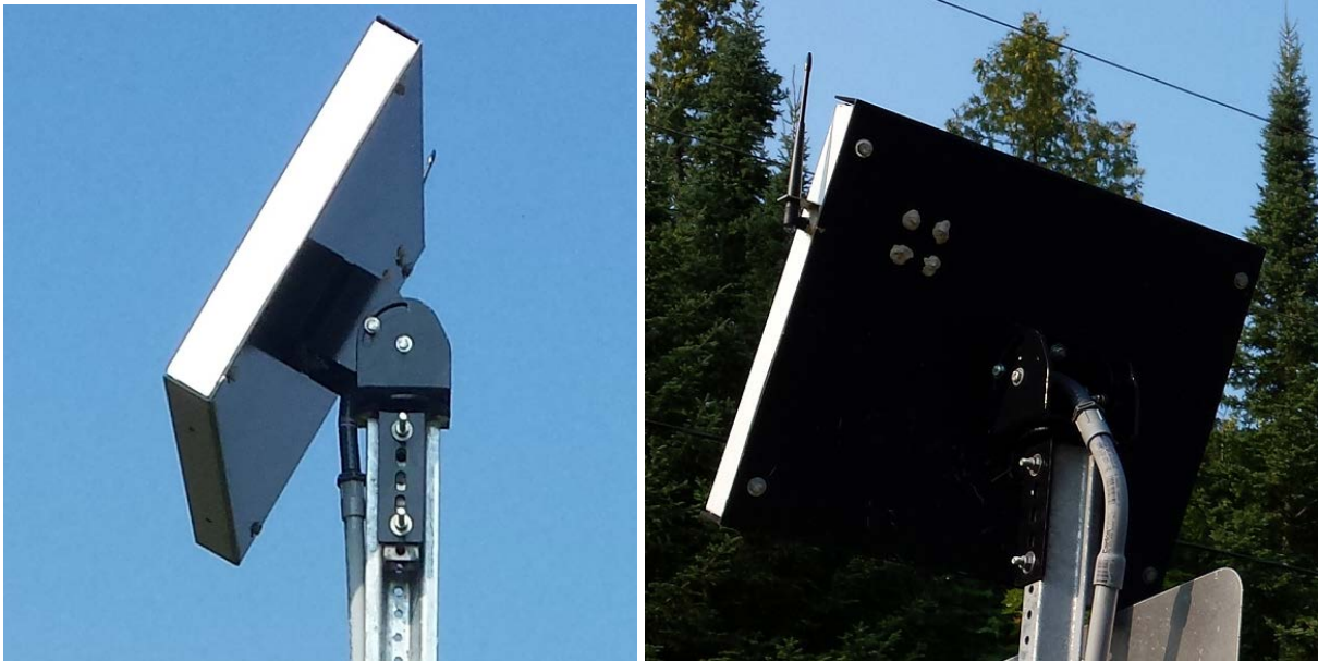
Figure 38: Solar panel housing and its mounting bracket.
