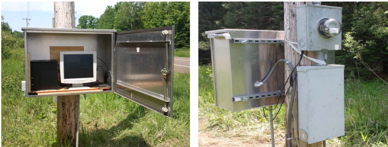
Figure 54: Data collection cabinet front view (left) and back view (right).
