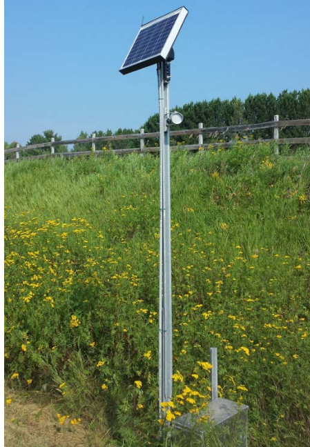
Figure 49: Installed Doppler radar unit (D2) on the major road.
