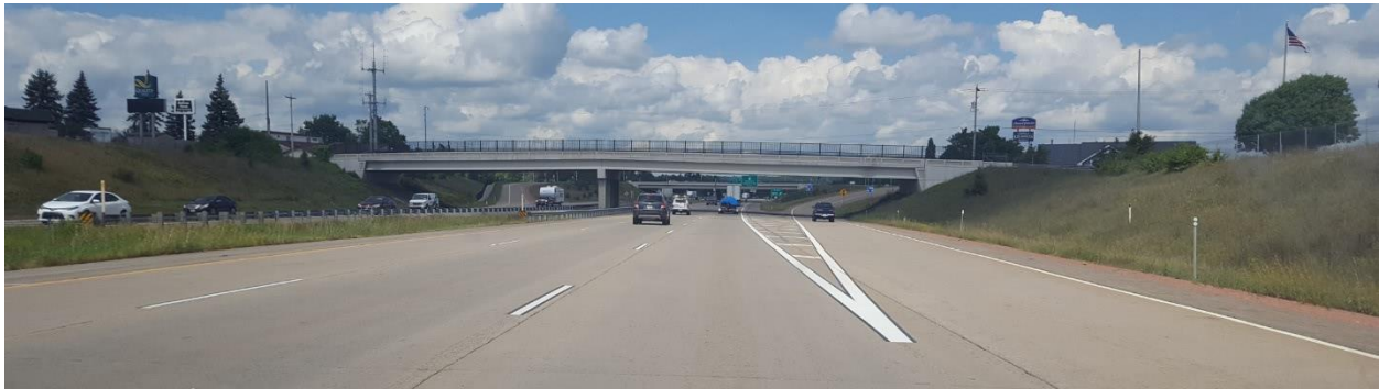
Figure 40: Bordered contrast markings on NB US-51
