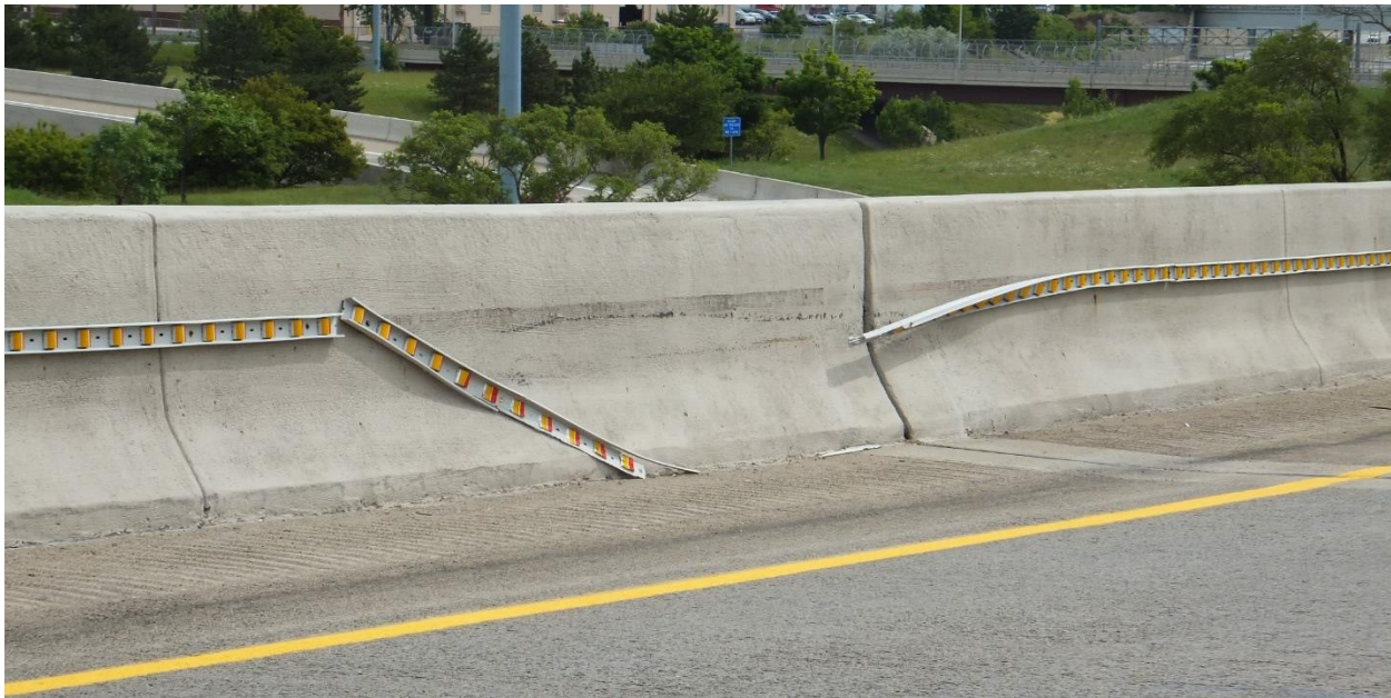
Figure 29: Damaged Luciol Systems Bi-directional reflector installed on barrier wall (Photo taken June 13, 2016. Opus International Consultants Inc.)
