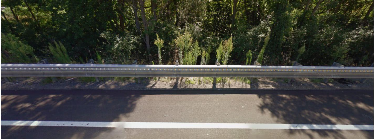
Figure 28: Luciol Systems Bi-directional reflector installed in guardrail channel (Image courtesy of Google Street View)
