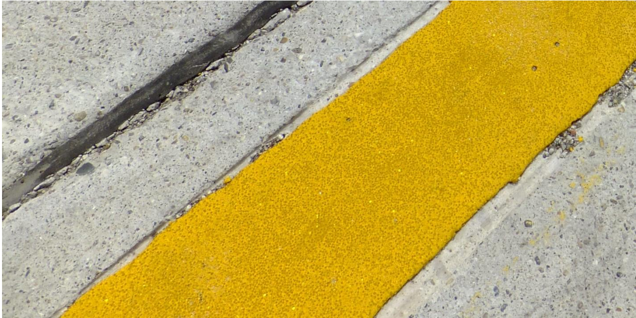
Figure 30: HPS-8 installation on Eton Road in Birmingham, Michigan (Photo taken June 13, 2016. Opus International Consultants Inc.)
