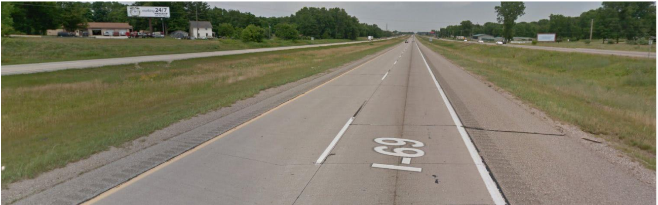
Figure 33: Contrast markings on NB I-69 (Image Courtesy of Google Street View)
