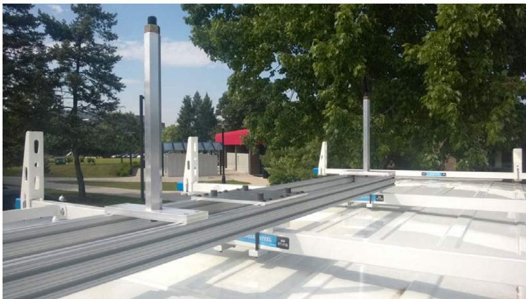
Figure 5 The Installed Sensor Mounting Platform
