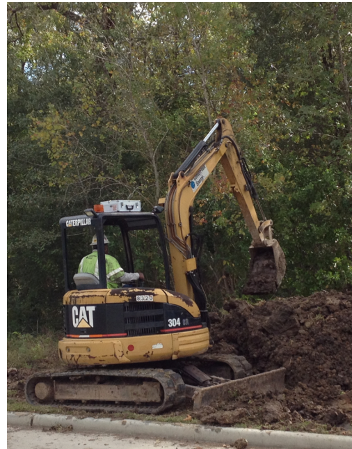
Figure 7: Hardware Components (Silver Briefcase), Installed on Centerpoint Energy Excavator for Testing – 11/20/2014.
