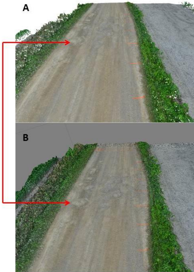
Figure 3-31: A comparison of the point clouds generated by the RSPS (A) and Agisoft PhotoScan which is a commercially available SfM software (B). The red line identifies the same pothole on each point cloud.
