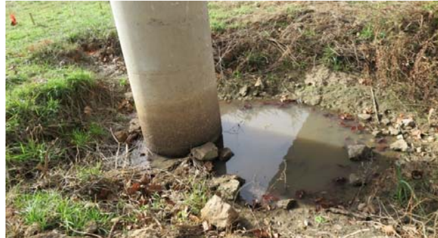
Figure 4.6. The bridge pier with a scour hole as a field test site.
