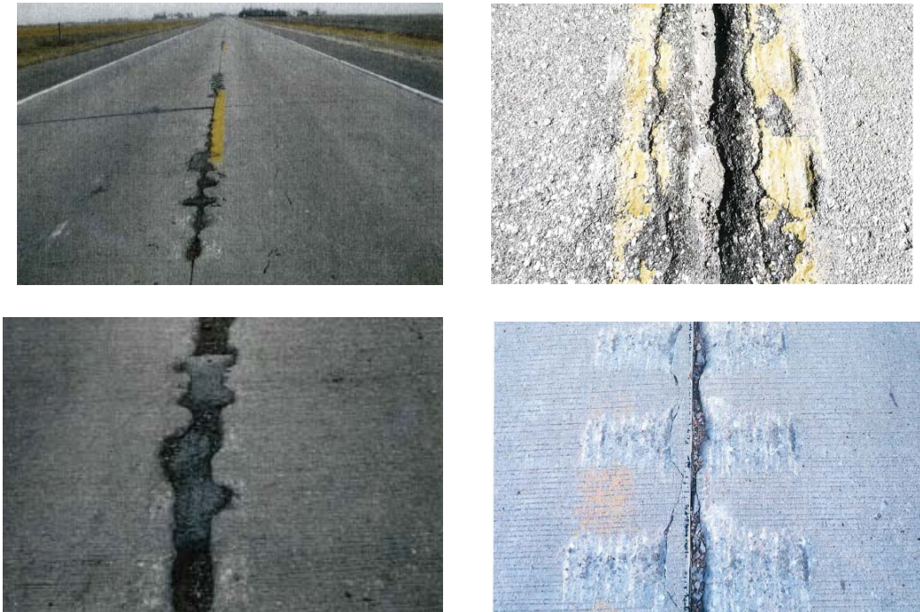
Figure 1-3. Pavement damage associated with CLRSs.
