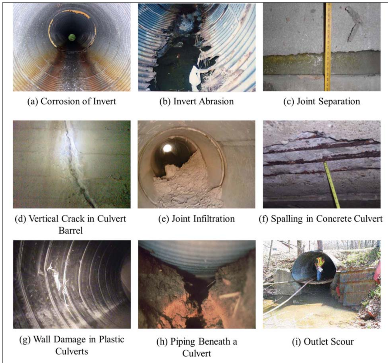
Figure 2. Common Defects Observed in Culverts
