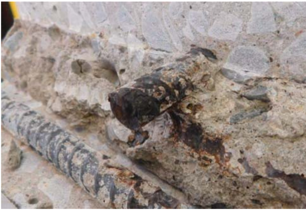
Figure 3.19 End of transverse bar exposed during uncracked specimen autopsy.
