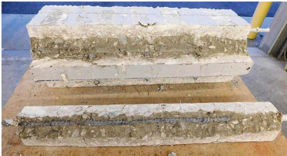
Figure 4.18 Specimen No. 42—damp interior of deck sealer specimen.
