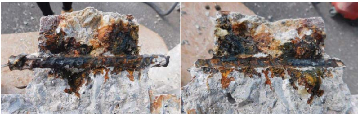
Figure 3.8 Corrosion product at crack interface.
