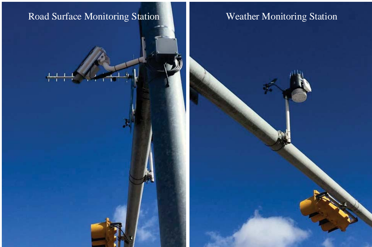
Figure 27. Weather and Road Surface Condition Monitoring Systems Deployed in Dumas, TX.
