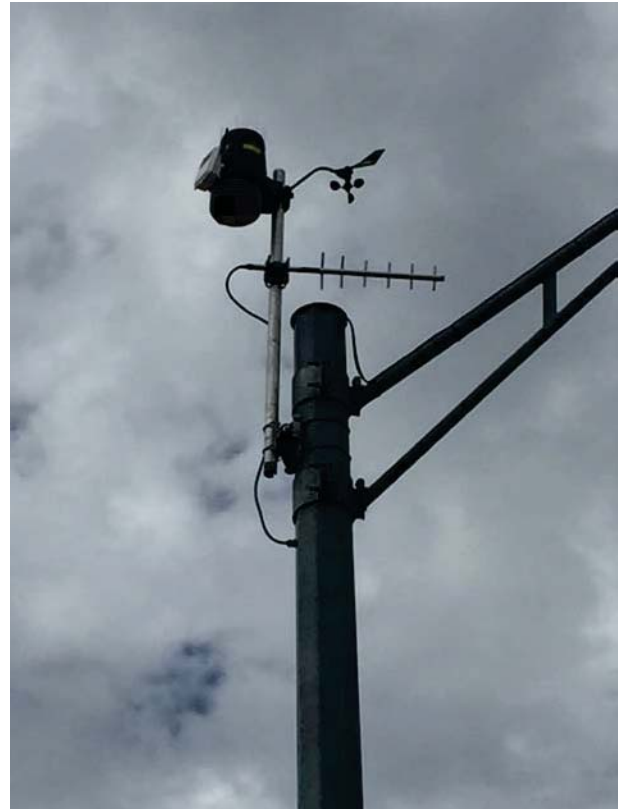
Weather Monitoring Station
