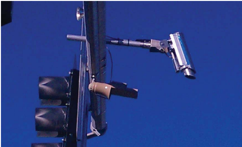
Figure 17. Typical Installation of Pavement Surface Monitoring Sensor – Off Signal Mast Arm.
