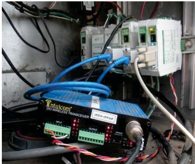
Figure 50. Image of Contact Closures and Radio.
