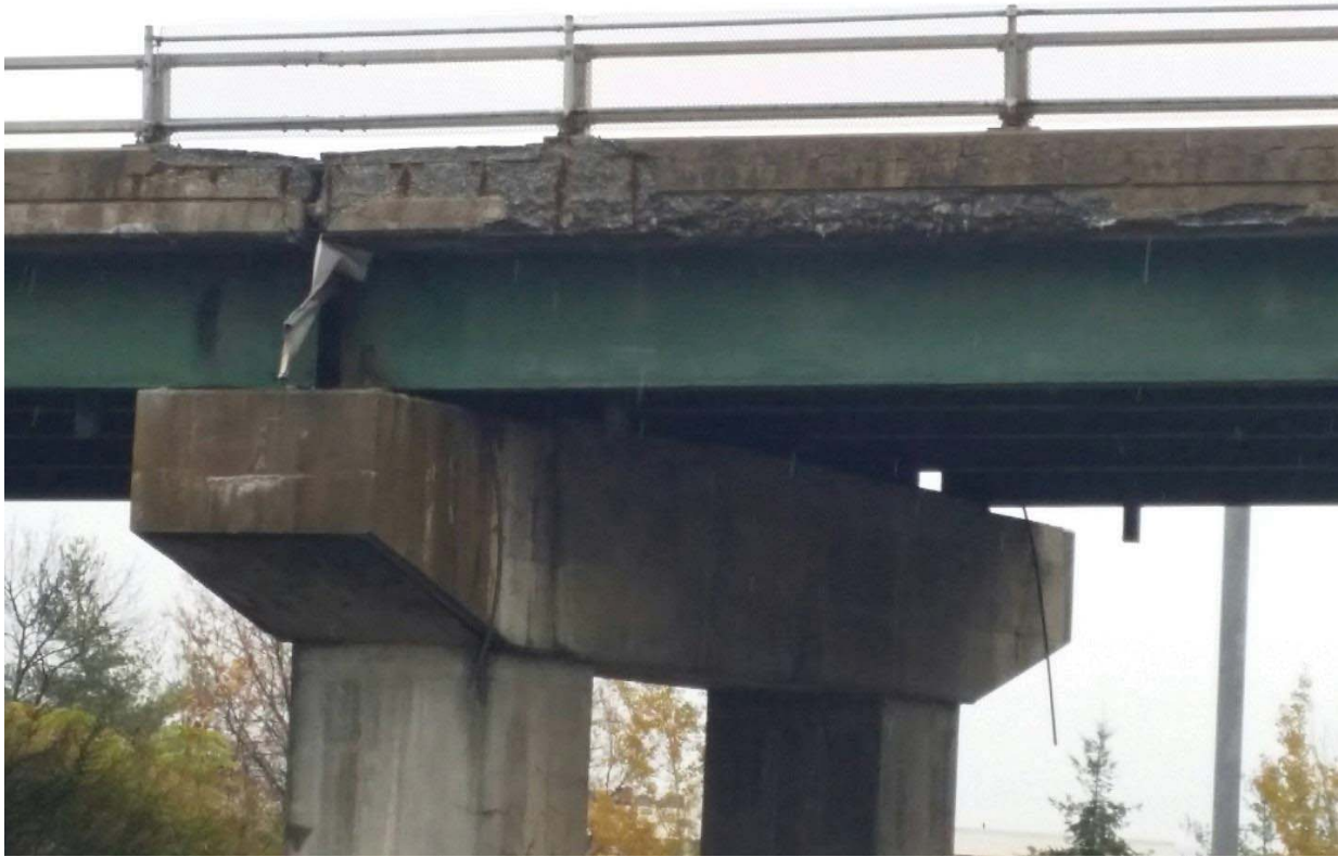
Figure 5.22 Closeup of Williston I-89 Overpass Tafts Corner with encasement repair of the pier, failed expansion joint gutter and distressed fascia
