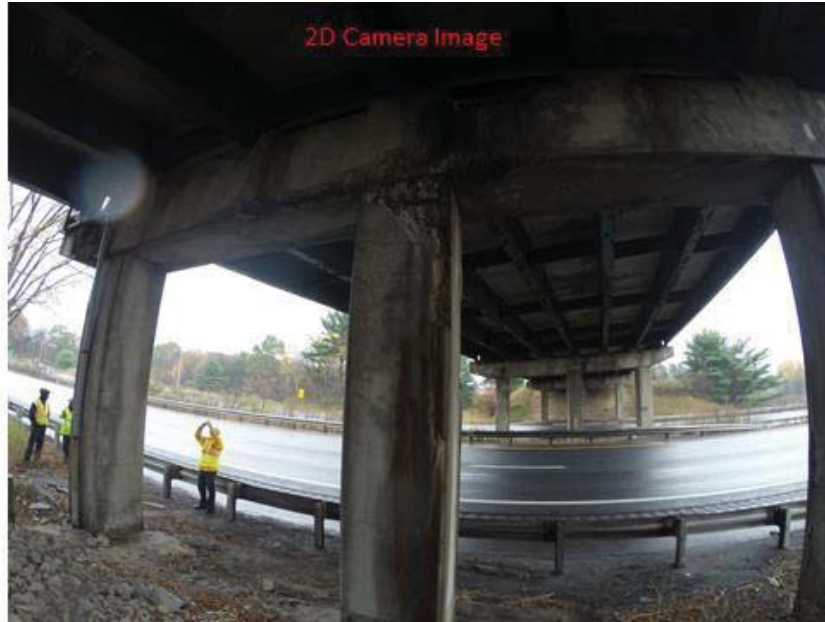
Figure 5.12 Spalling on column of Colchester/Milton I-89 Bridge
