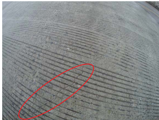
Figure 37: Crack on Deck Surface. Highlighted by Red Oval
