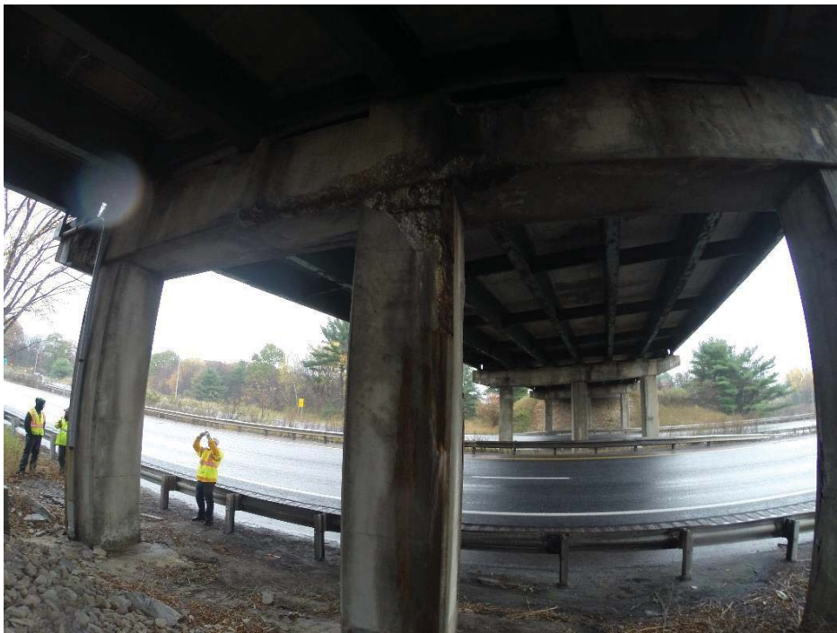
Figure 19: Column and cap Spalling and steel corrosion
