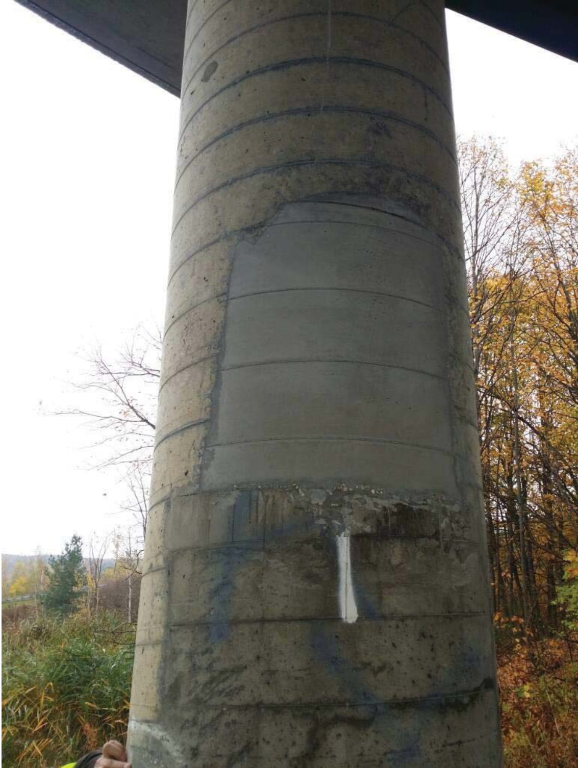
Figure 5.24 Small column patch repair #2 on Williston I-89 Oak Hill Rd Underpass Bridge
