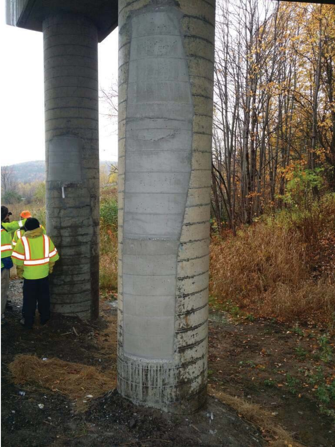
Figure 5.25 Large column patch repair #1 on Williston I-89 Oak Hill Rd Underpass Bridge
