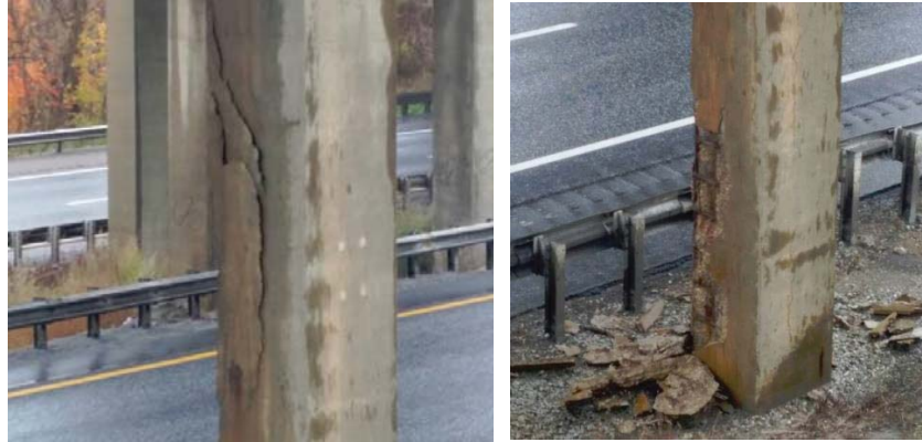
Figure 33: Spalling and steel corrosion on concrete column. Notice concrete fragments falling near road.
