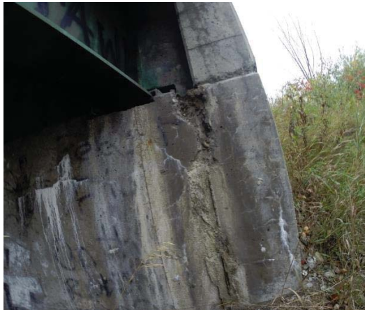
Figure 29: Scaling on abutment around bearing and beam
