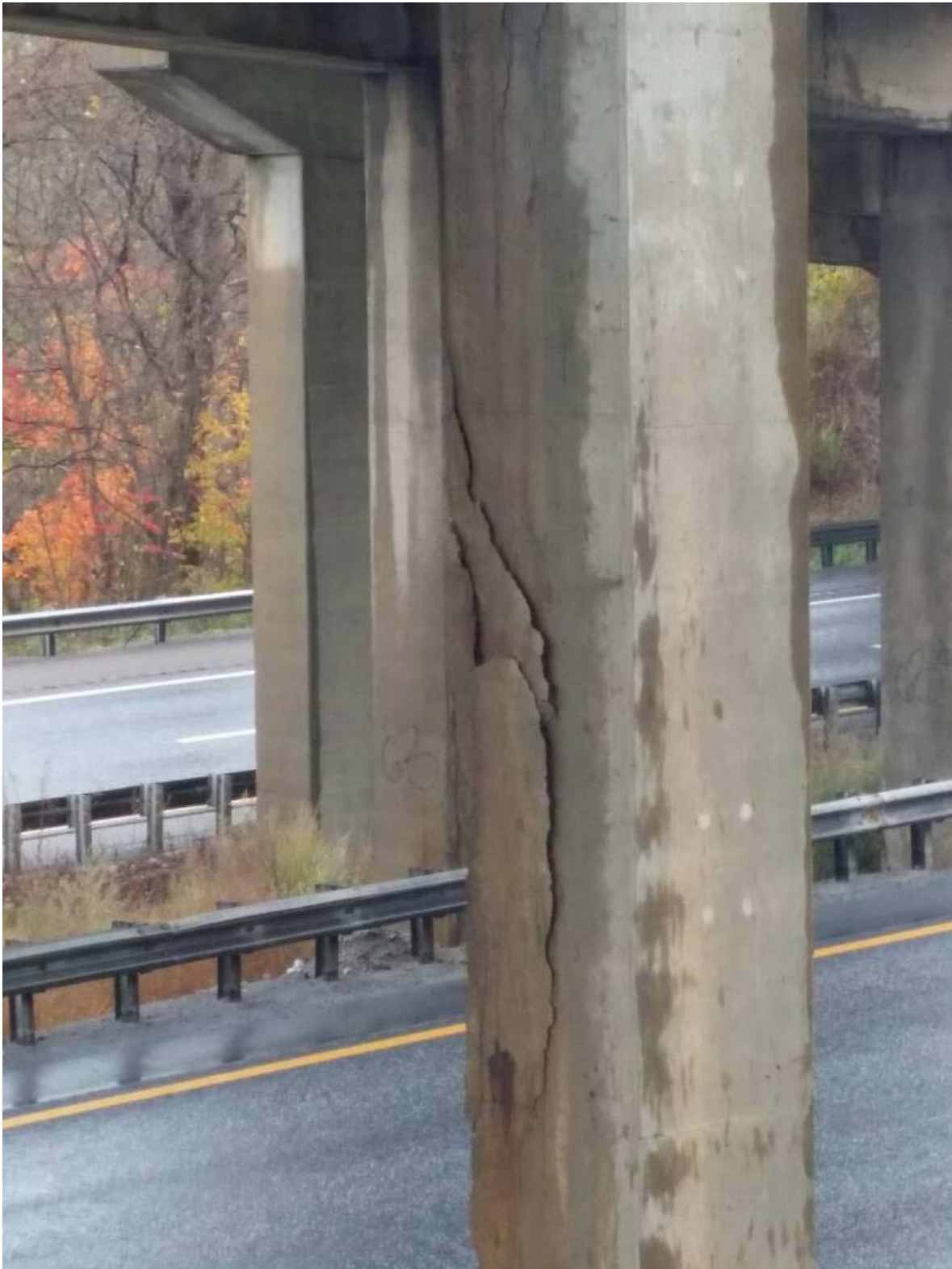
Figure 5.35 Column with spalling at the corners on Richmond I 89 US 2 Underpass Bridge
