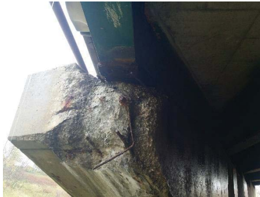
Figure 34: End cap spalling and steel corrosion with non-existing bearing.
