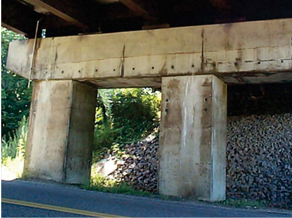
Figure 5.20 Spear St. I 189 Overpass Bridge pier in 2000 recently encased, with cracks
