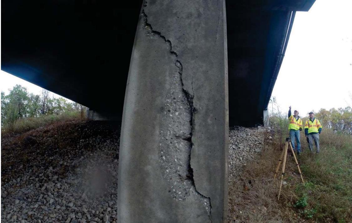
Figure 5.14 Column with distress on Colchester/Milton I-89 Bridge
