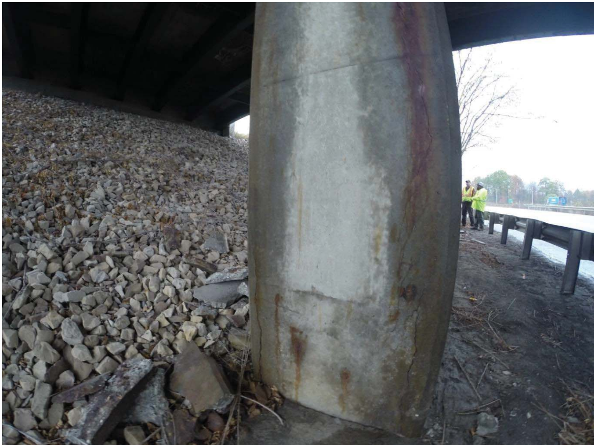
Figure 5.9 Column on Colchester/Milton I-89 Bridge showing cracking, likely due to swelling corroded reinforcing bars
