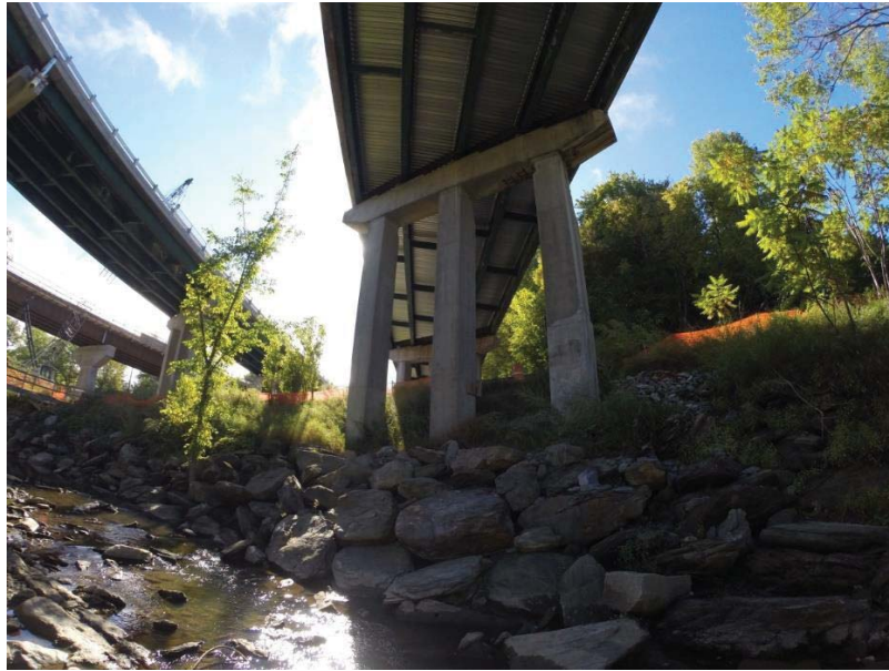
Figure 5.52 Repaired pier on I-89 Waterbury Overpass Bridge with patch repairs, note the use of integrated corrugated panels on new concrete deck.
