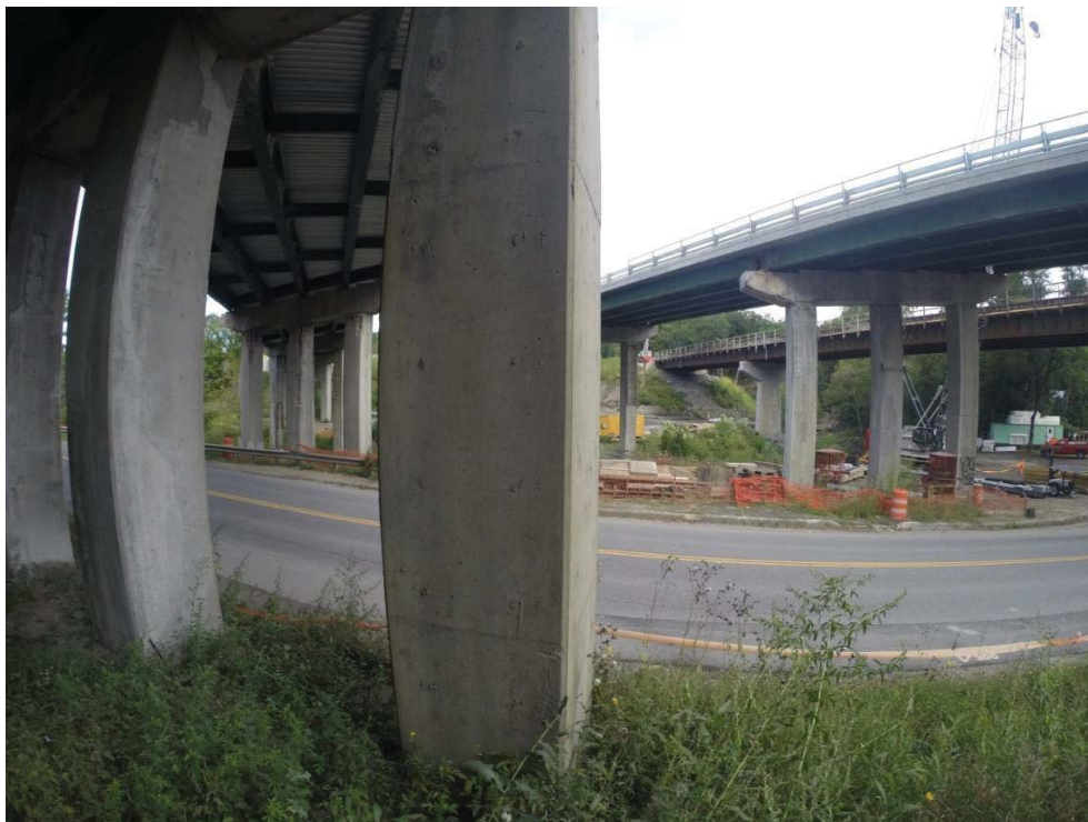
Figure 5.51 Pier on I-89 Waterbury Overpass Bridge with patch repairs
