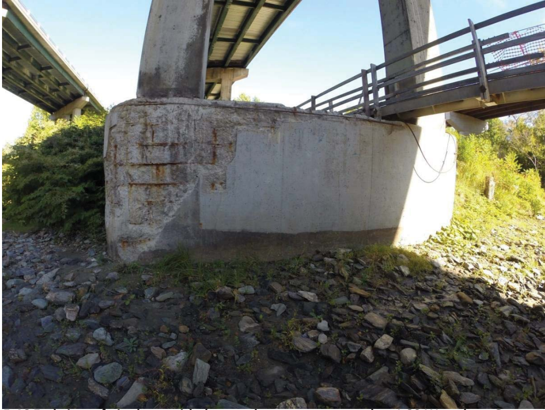
Figure 5.46 End view of pier base with damaged concrete removed on I-89 Waterbury Overpass Bridge
