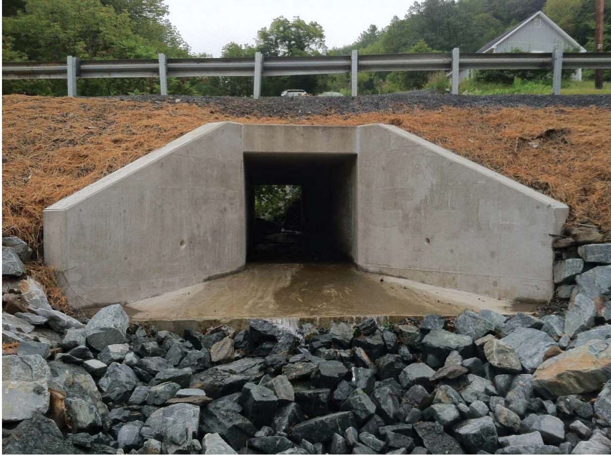
Figure 4.32 Vt.Rte.14 Hartford Br.#7 - REPAIRED Wing Wall/ Cut-off Wall Reconstruction $180,000
