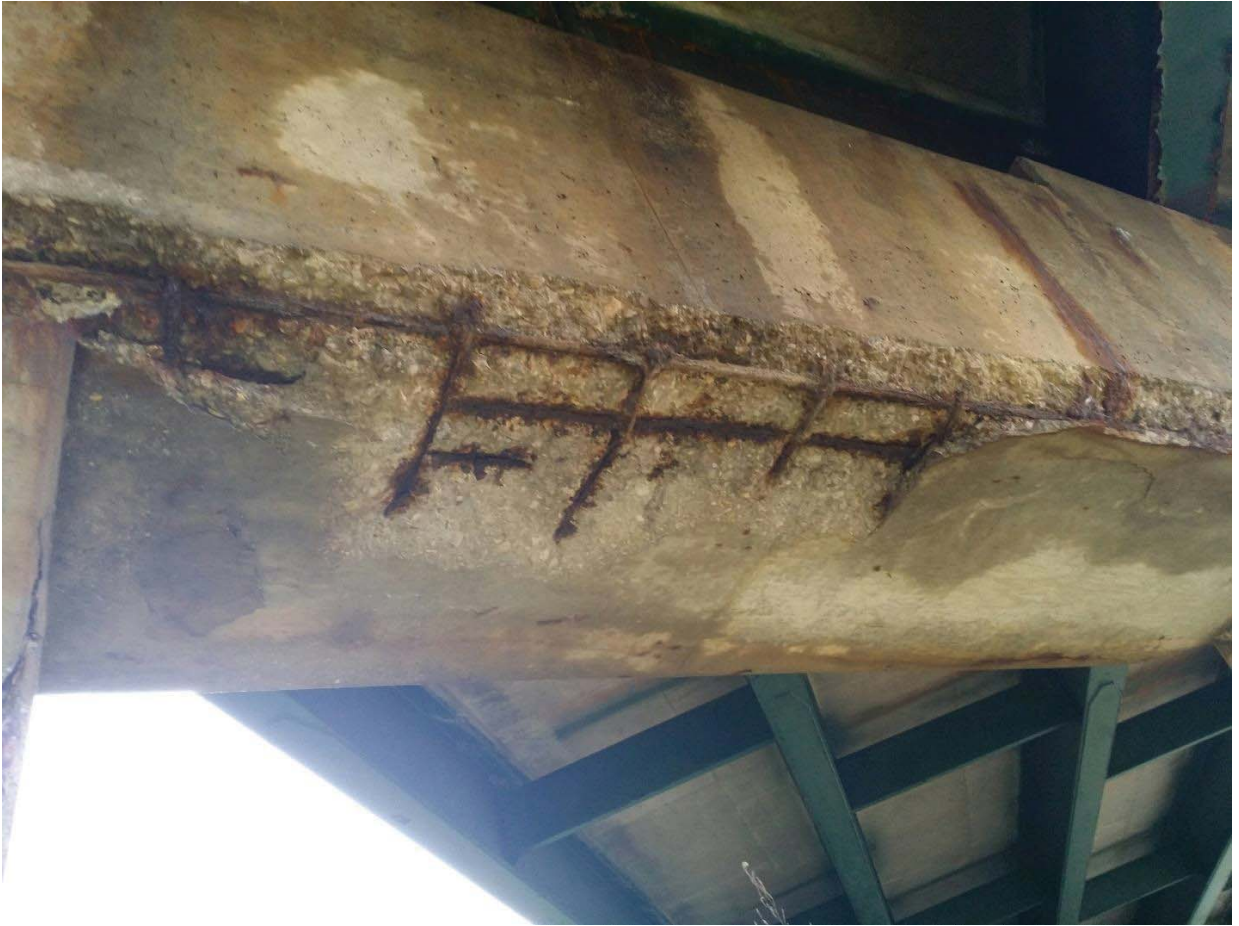
Figure 5.32 Pier cap with spalling on Richmond I 89 US 2 Underpass Bridge
