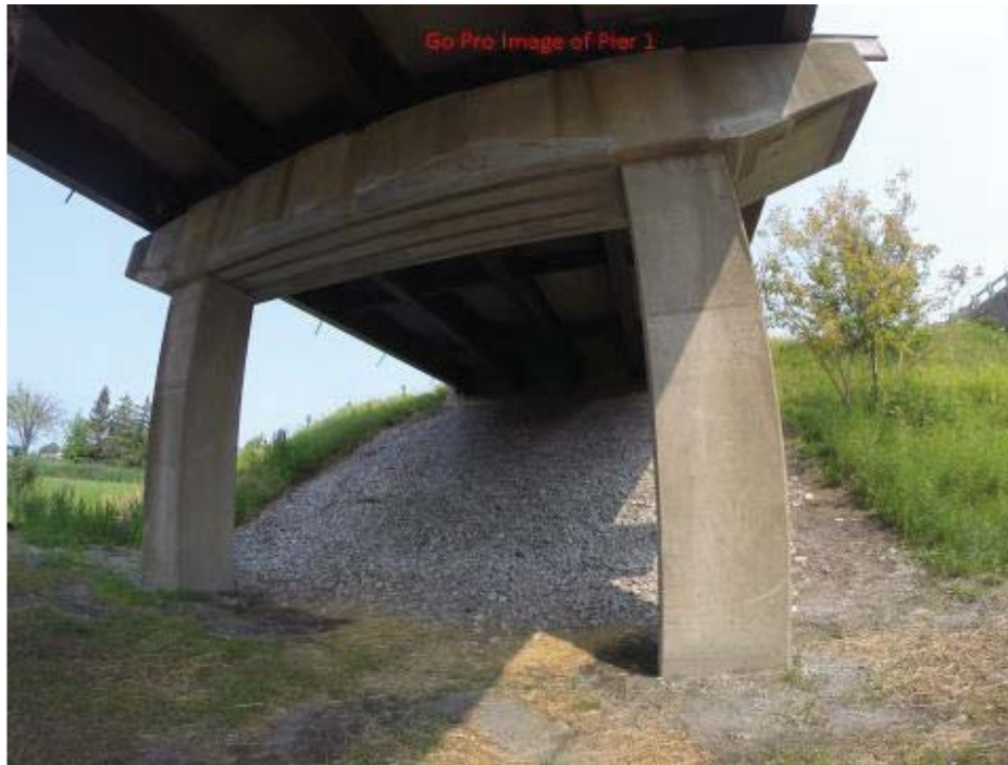
Figure 5.1 Swanton I 89 overpass bridge with FRP strengthening strips bonded to the piercap
