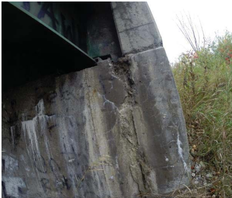
Figure 5.28 Scaling on Abutment and Beam on Williston I-89 Oak Hill Rd Underpass Bridge
