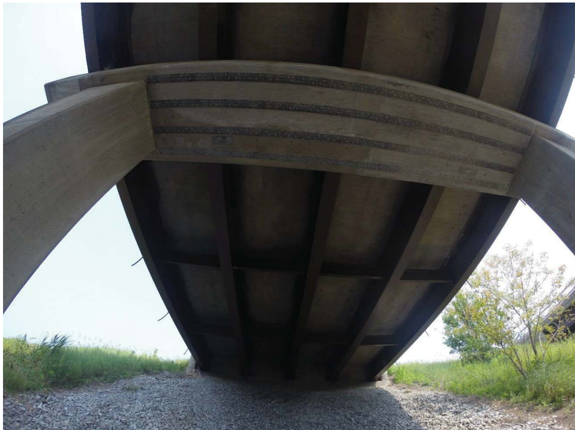
Figure 5.2 Swanton I 89 overpass bridge with FRP strengthening strips bonded to the pier cap, bonding bolt pattern is discernible.
