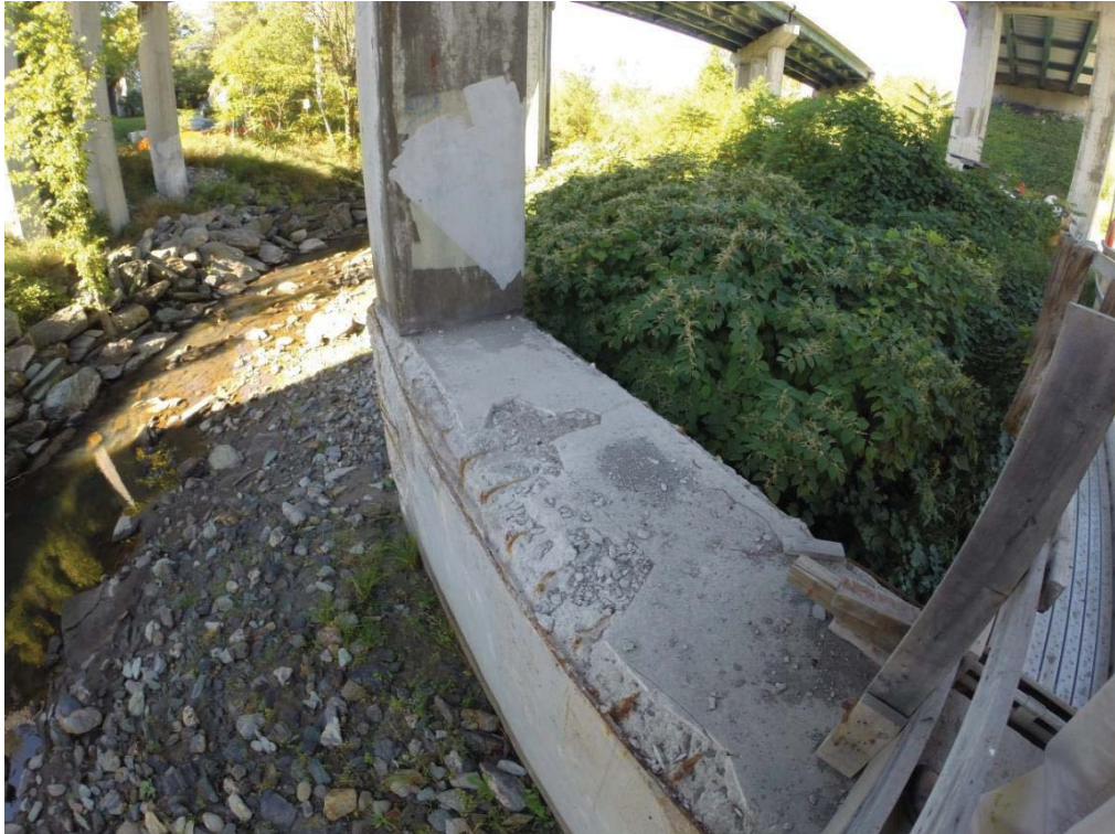
Figure 5.47 Top view of pier base with damaged concrete removed on I-89 Waterbury Overpass Bridge
