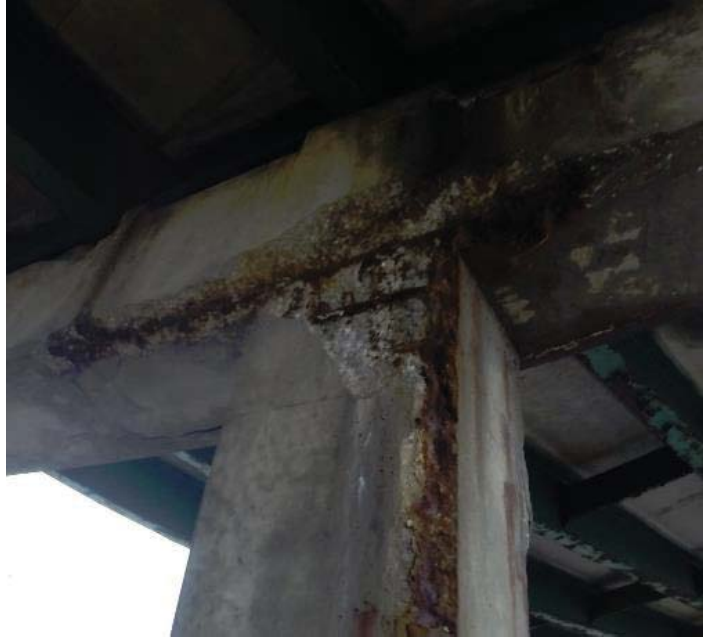
Figure 20: Close-up of concrete spalling and steel corrosion on middle column and cap
