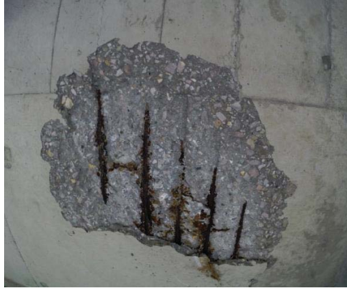
Figure 30: Spalling and slight steel reinforcement corrosion on underneath portion of concrete deck
