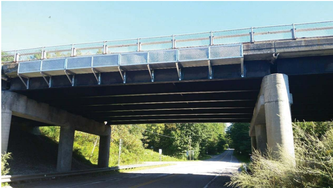
Figure 5.53 I 89 Middlesex Overpass Bridge with supplemental rack to protect vehicles passing under by catching pieces of concrete that spall and fall from the fascia
