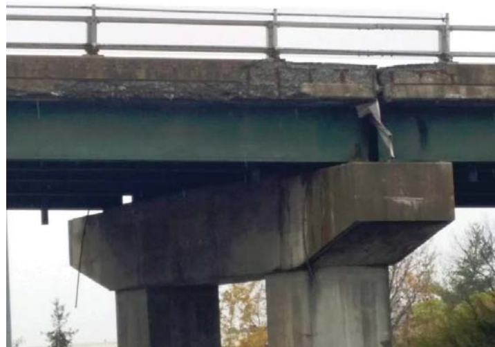
Figure 27: Spalling and steel corrosion on concrete fascia.
