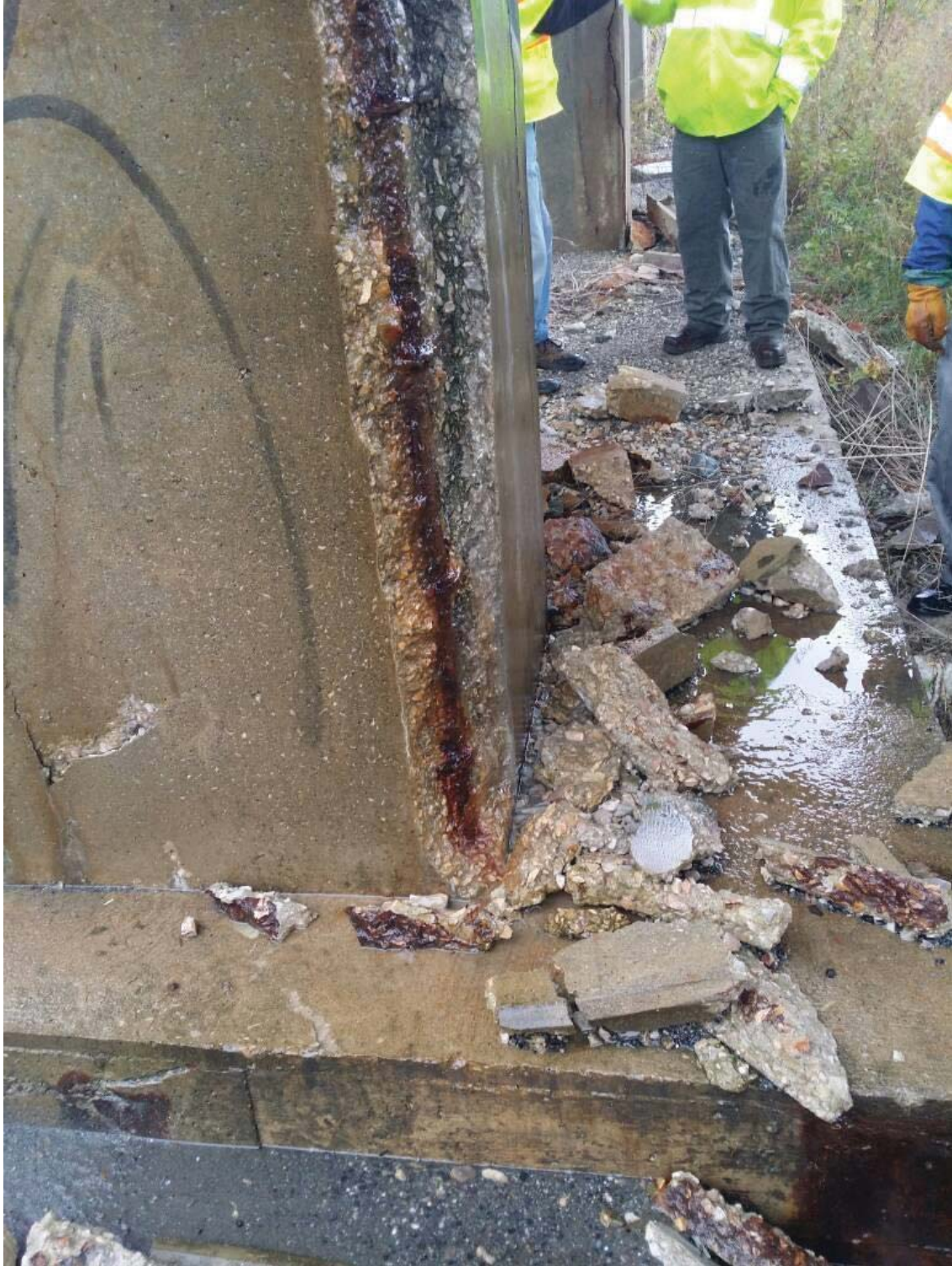
Figure 5.33 Square column with spalling at the corners on Richmond I-89 US 2 Underpass Bridge
