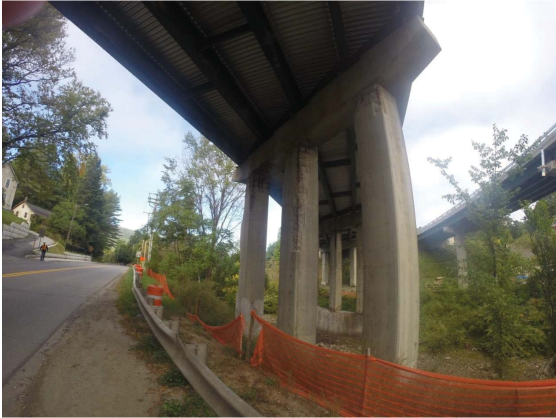
Figure 5.48 Pier on I-89 Waterbury Overpass Bridge with corners prepared for patch repairs
