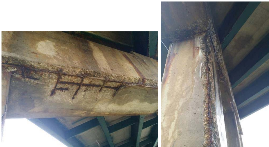
Figure 32: Spalling and steel corrosion on columns and caps
