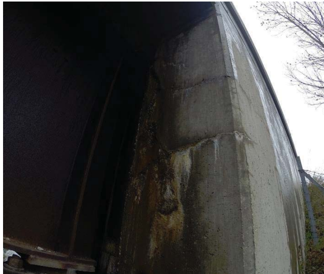
Figure 25: Scaling and cracking on abutment. Corrosion stains from steel beams
