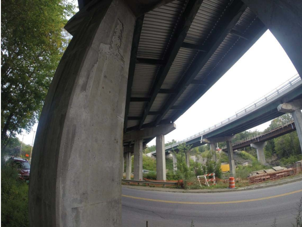
Figure 5.50 Pier on I-89 Waterbury Overpass Bridge with patch repairs, note the extended gutters on span in background
