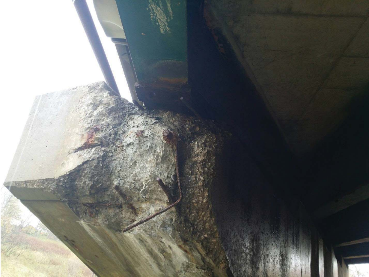
Figure 5.38 Close-up of pier cap with lost corner section leading to subsided bearing on Richmond I 89 US 2 Underpass Bridge
