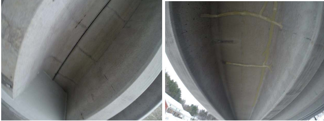
Figure 38: Underside of Concrete Deck. Left Image: chows cracks going at the way through concrete deck. Cracks are highlighted by red ovals. Right Image: sealant used to seal large cracks.
