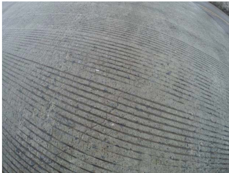
Figure 5.42 Deck patterned with cross-span cracks, approximately every 200 mm on Stowe Rte 100 Gold Brook Crossing Bridge
