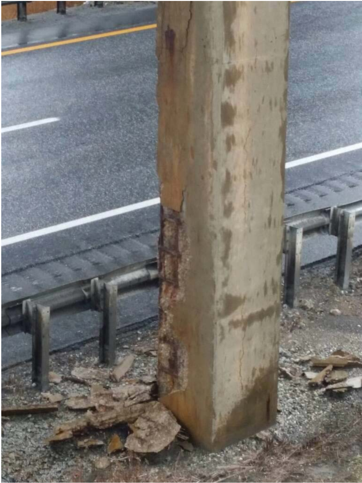
Figure 5.36 Column with spalling at the corners and side on Richmond I 89 US 2 Underpass Bridge
