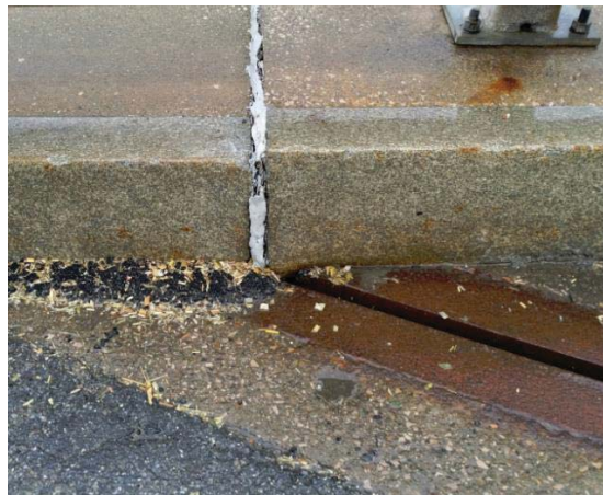
Figure 35: Bridge deck and expansion joint. Because of non-existing bearing bridge deck has settled down about 1.5”.
