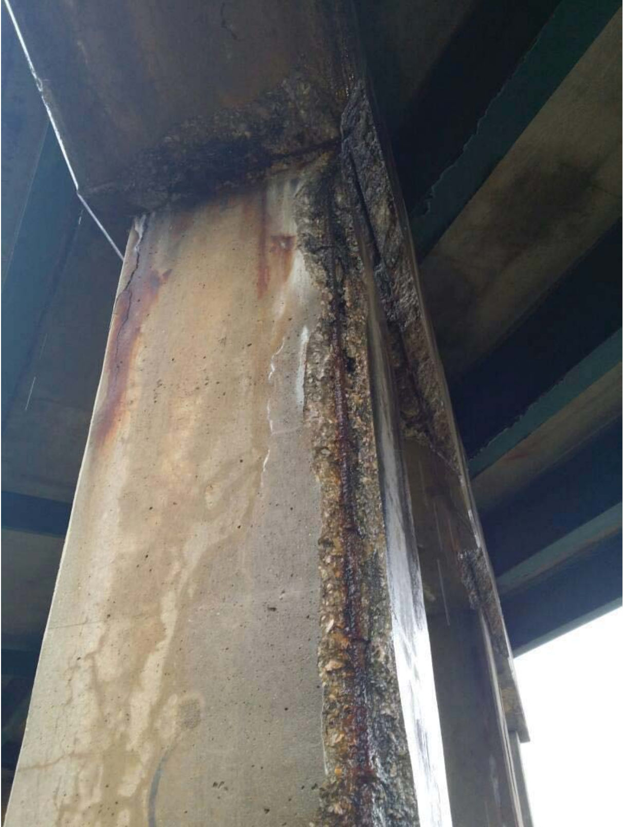
Figure 5.34 Square column with spalling at the corners and pier cap on Richmond I-89 US 2 Underpass Bridge
