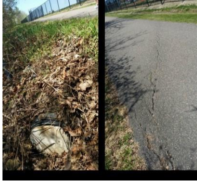
Figure 57 (a) Test Spot Plugged with Concrete Drain Pipe; (b) Asphalt Pavement Crack on the Surface
