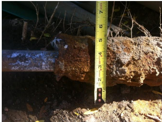
Figure 43 An excavated pipe which was consistent with the GPR result in Figure 34
