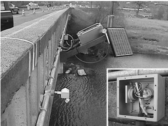
(a) An installed tiltmeter
