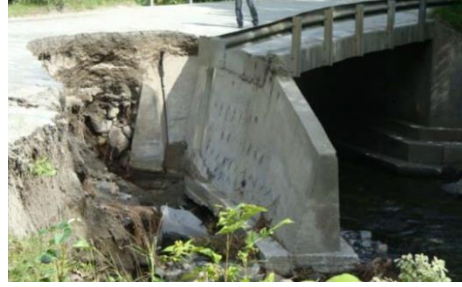
Approach scour (Orleans, Vermont)
