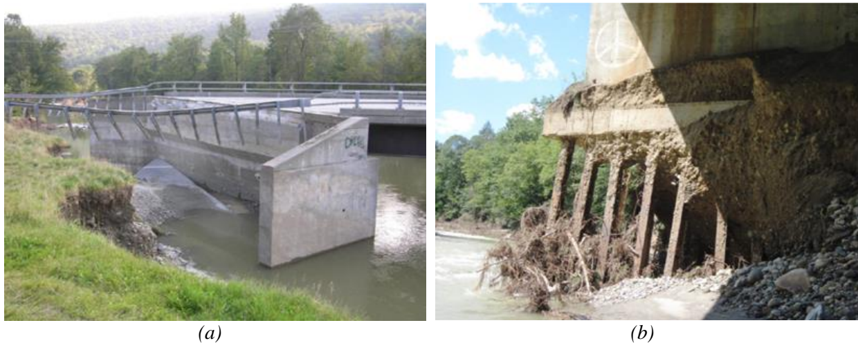
Figure 6.3: Example of flanking (a) and abutment scour (b) damage to bridge embankment and abutment due to Tropical Storm Irene (source: Vermont Agency of Transportation, 2014)
