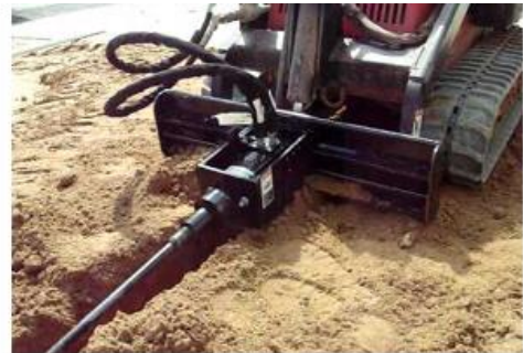
Figure 28. Cost of cleaning drains ($/LF) using a skid steer HDD drill with rotowitch & Harr tools
