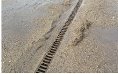
Figure 10- Debris cleaned from the drain
