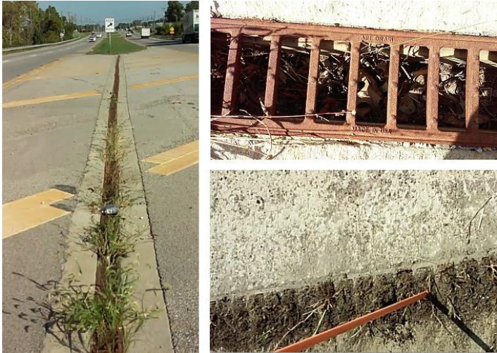
Figure 3- Debris and vegetation in trench drains
