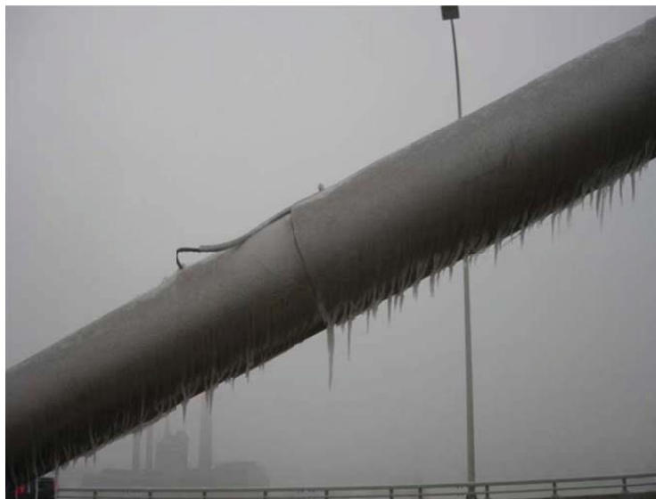
Figure 1.3: Ice Accumulation on the East Side of VGCS (Baker, 2007)
