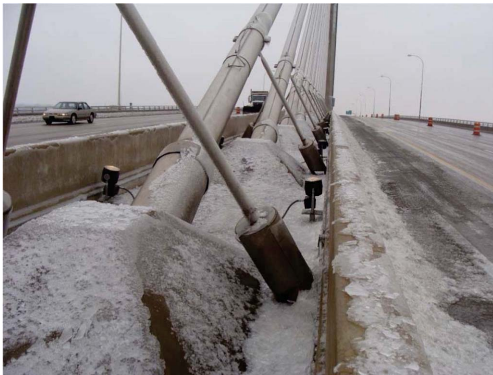
Figure 1.20: Ice on bridge deck after 80-90% had shed, February 24, 2011
