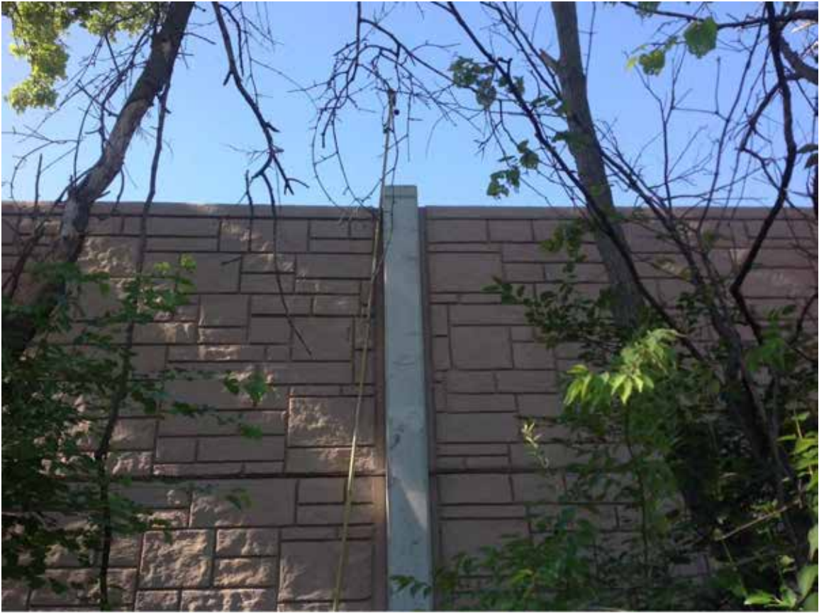
Site 15: FRA-70 WB, Bellow Falls Pl, Looking at Meter A
