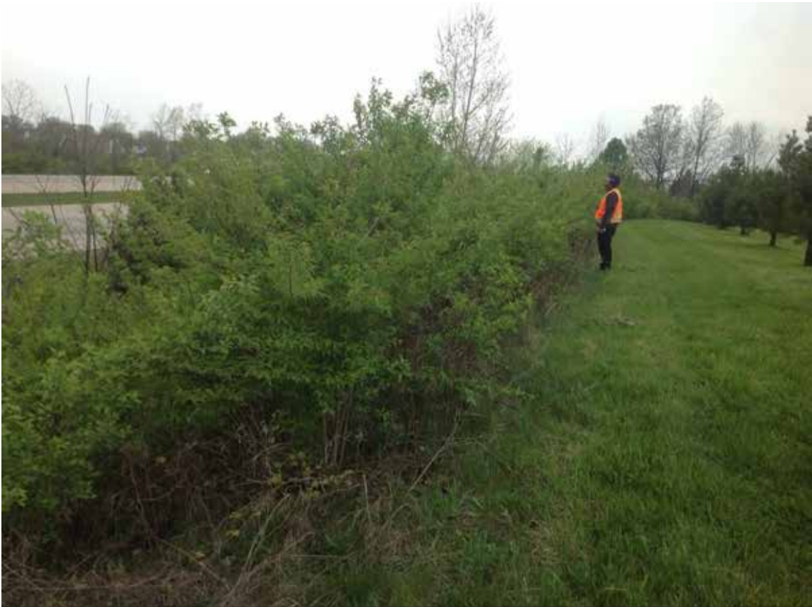
Site 24: FRA -270 WB, Exemplar Ct (Between Alkire and Big Run Rd), Looking along Noise Berm Southern Slope
