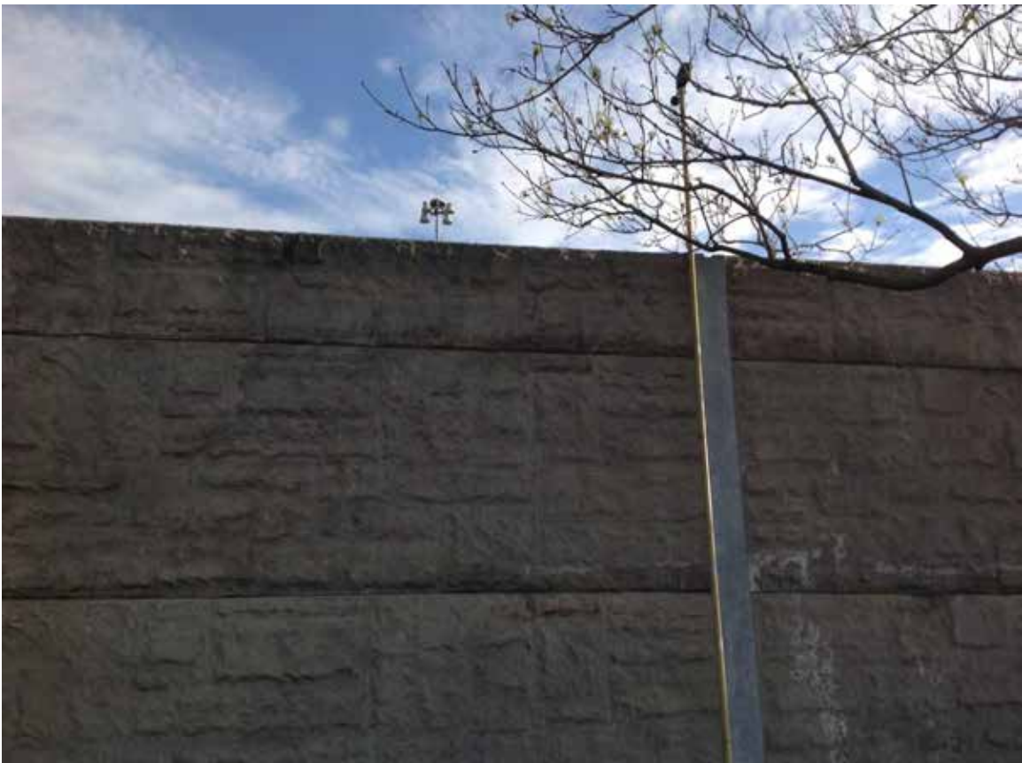
Site 19: CUY-480 WB, Preston Rd & Portland Rd, Looking at Meter A
