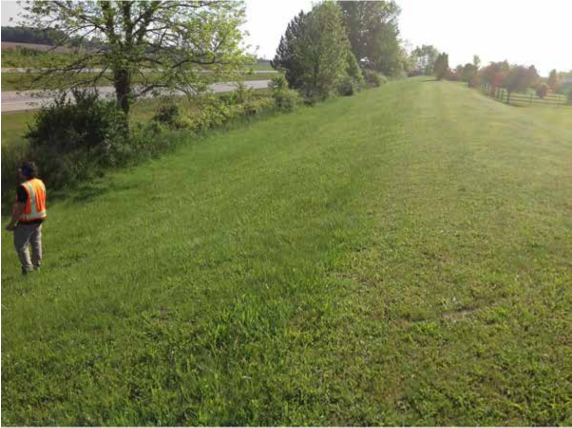
Site 34: CLI-71 NB, Jesse Drive Community, Looking along Noise Berm Western Slope
