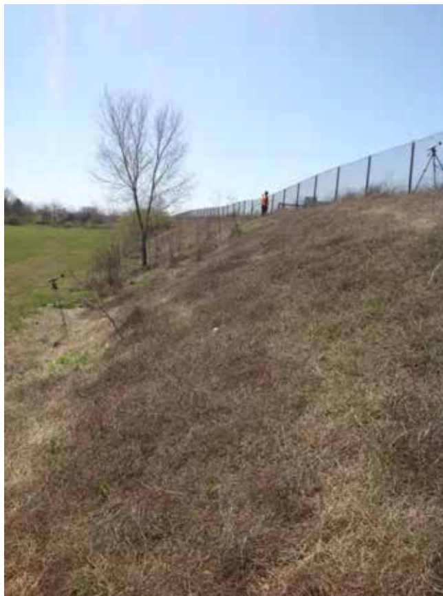
Site 14: MIA-75 NB, Swailes Road (Driving Range), Looking along Noise Berm Western Slope
