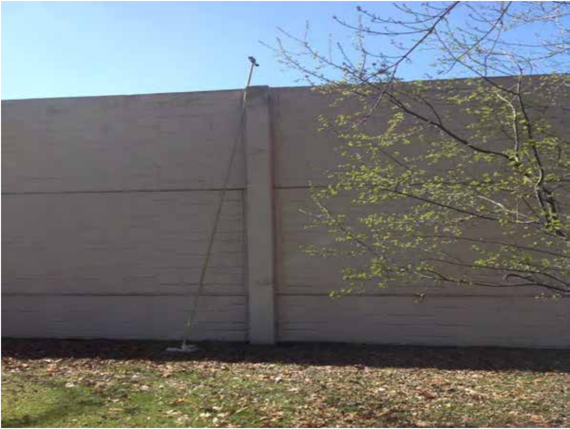
Site 7: LUC-475 SB, Seccor Rd (Sisters of Notre Dame), Looking at Structural Wall
