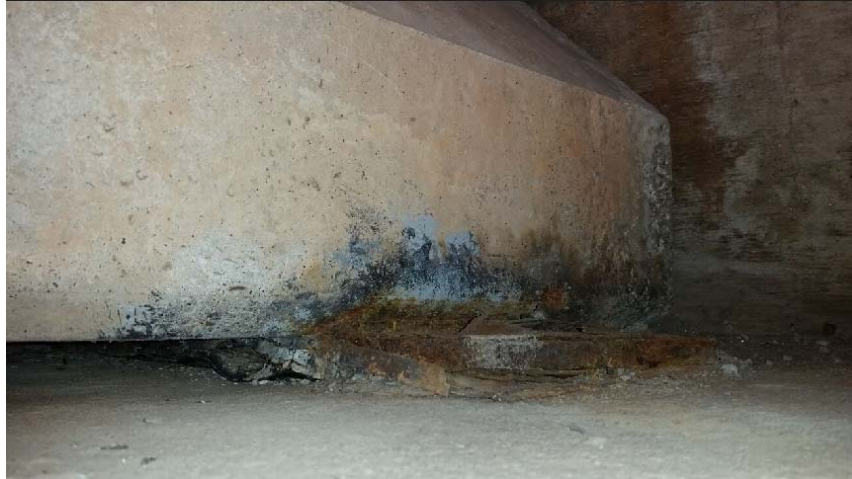
Figure D-29: Corroded bearing plate and spalling along bottom of girder and girder end (3S-W)
