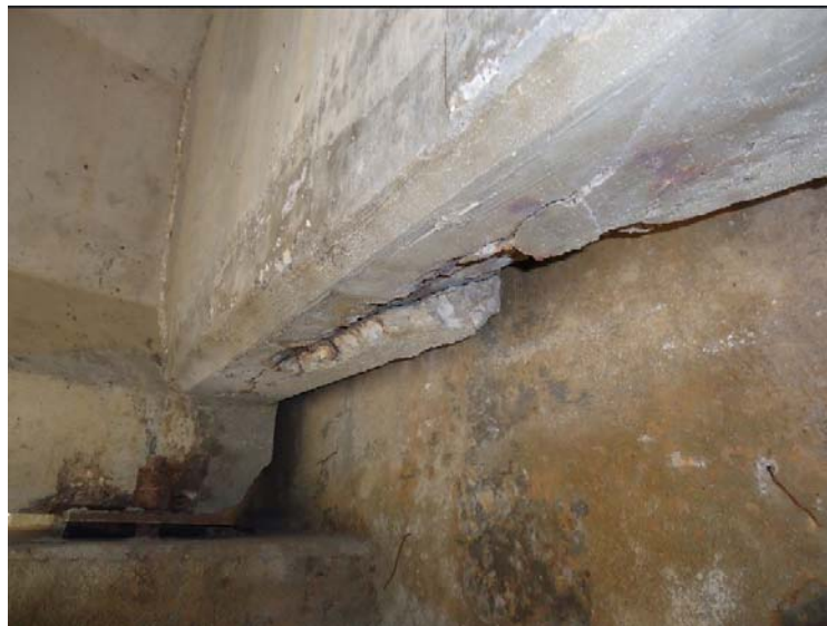
Figure D-15: Deterioration of an interior end diaphragm (6W-N); the diaphragm connects two interior beam ends
