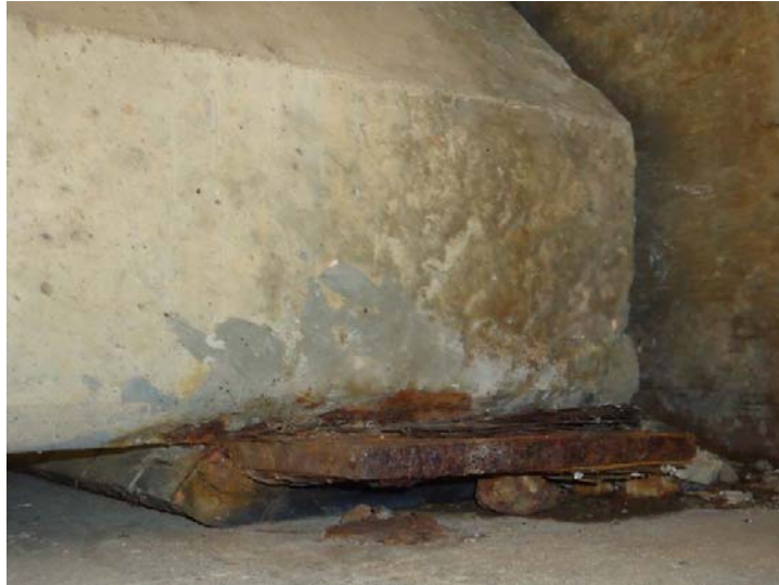
Figure D-35: Spalling above corroded bearing plate and missing anchor bolt (10E-S)
