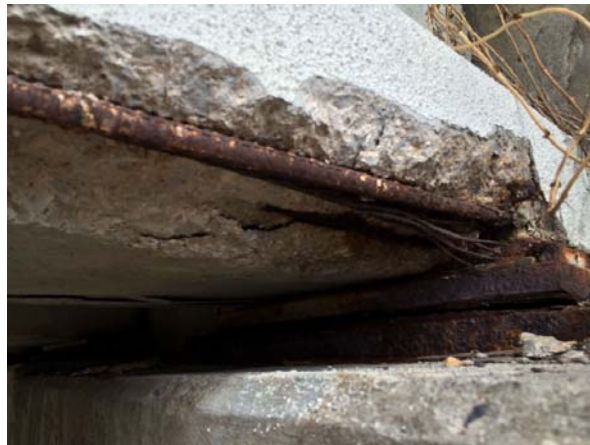
Figure 9-11: Example of exposed reinforcing steel
