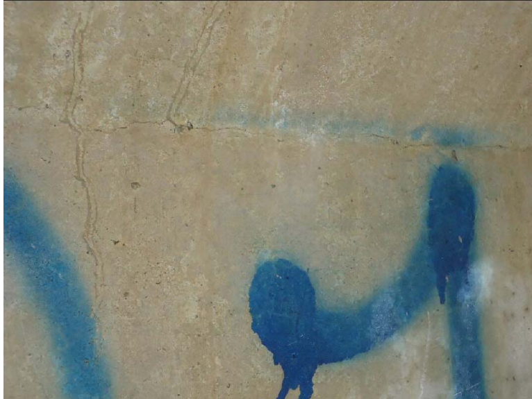
Figure D-61: Horizontal crack at top flange and web interface extending approximately one foot into the beam (1S-E)
