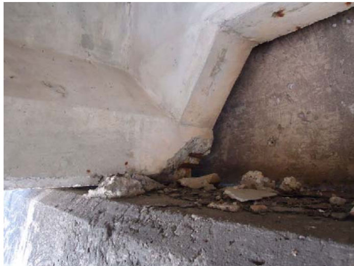
Figure D-70: Diagonal back corner spalling of diaphragm and exposed prestressing strands (5S-W)
