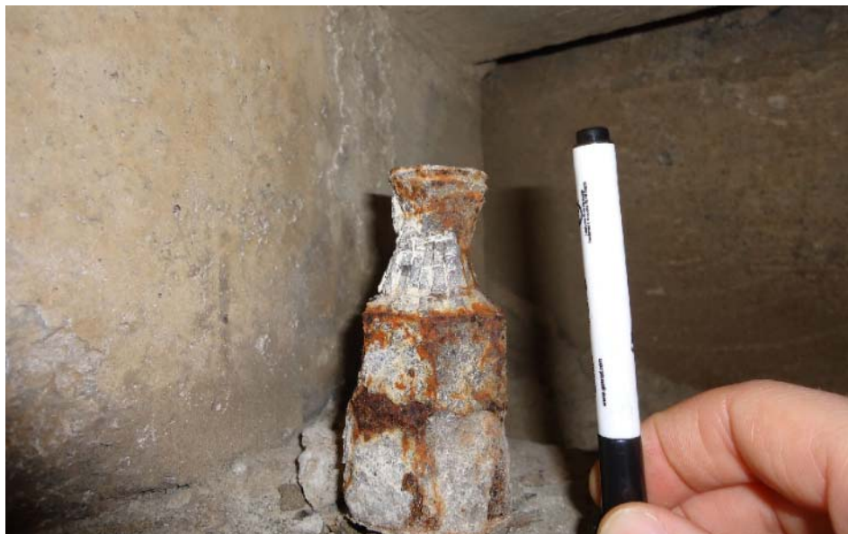
Figure D-17: Close-up of deterioration of anchor bolt, with necking at the top (4E-S). The pen is shown in the picture to illustrate the amount of necking occurring to the steel member.
