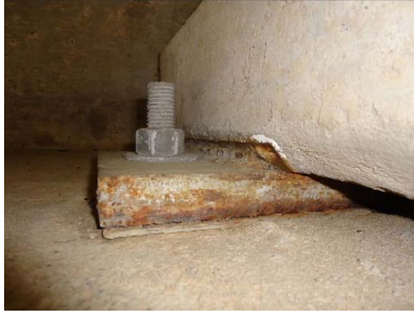
Figure D-2: Example of a corroding bearing plate (3W-S)
