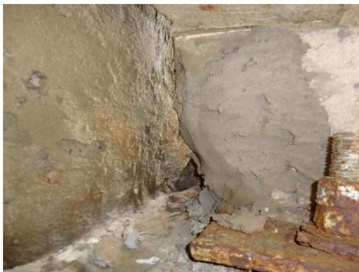
Figure D-9: Repair to spalled back corner (6N-W)
