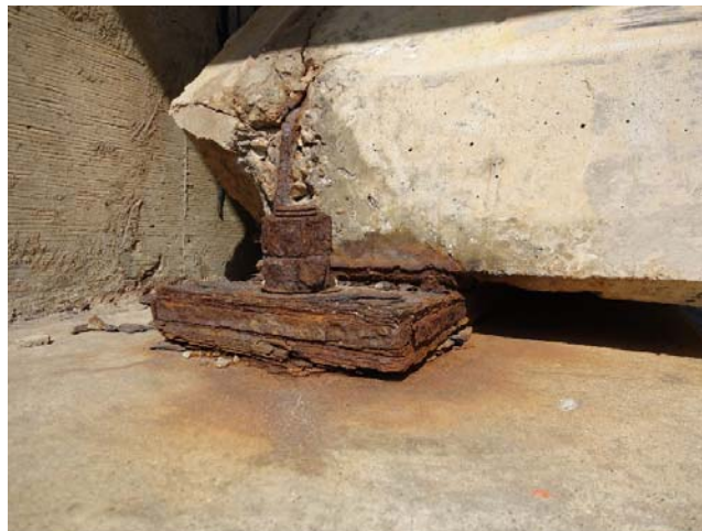
Figure 9-6: Example of corroded bearing plate
