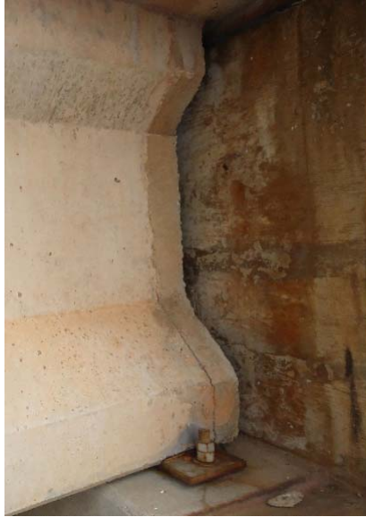
Figure D-47: Vertical separation of diaphragm and girder at interface (5E-S)
