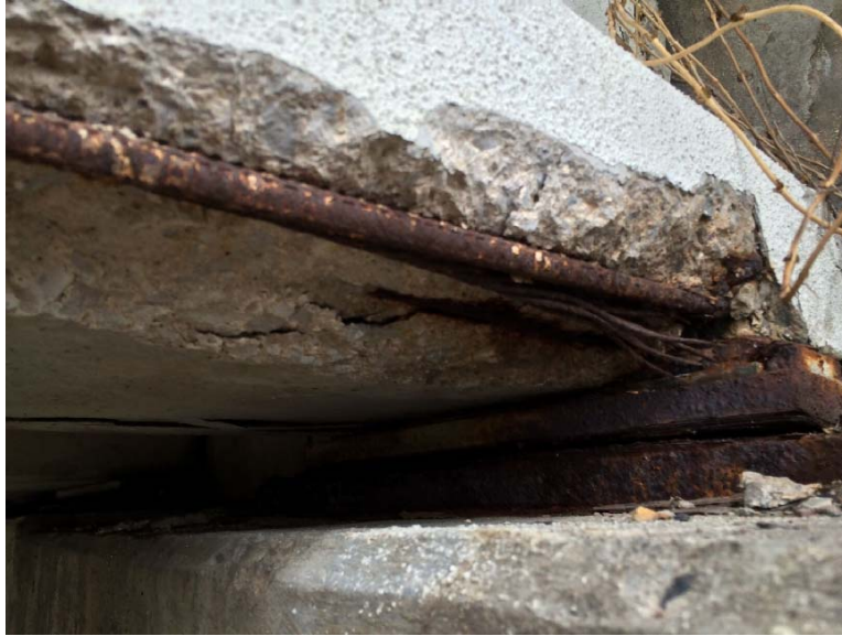
Figure D-23: Exposed rebar due to spalled concrete on the bottom of an exposed, exterior girder (1N-E)
