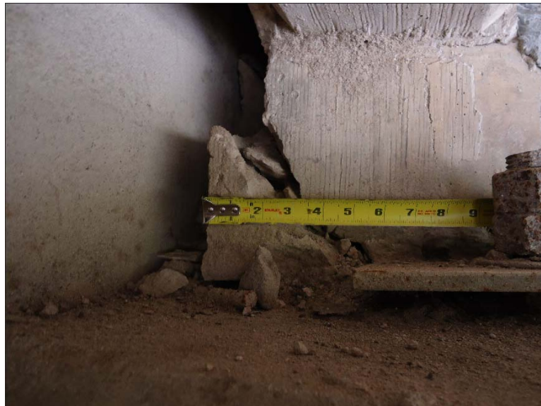
Figure D-13: Spalled back corner of beam end (4E-N)
