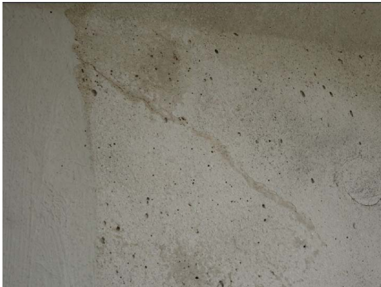
Figure D-38: Diagonal crack in web from top flange towards bottom of beam (1N-W)
