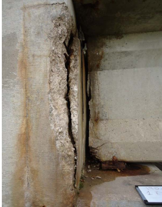
Figure D-31: Deterioration of back wall and girder end due to moisture/water (1E-N). The exposed, exterior girder has a corroded bearing plate and spalling occurring at the end.
