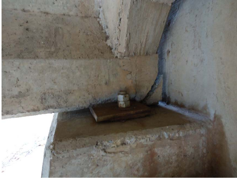
Figure D-45: Back corner diagonal cracking of exterior beam (1E-S)
