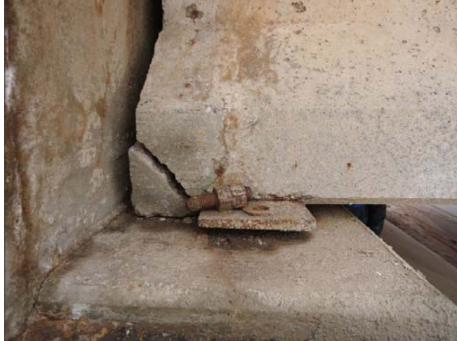
Figure D-43: Back corner diagonal crack of exposed, exterior beam (1E-N)
