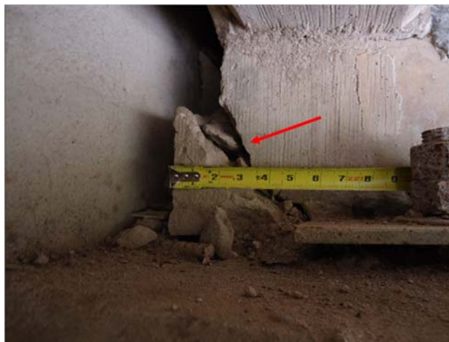
Figure 9-13: Example of back diagonal cracking
