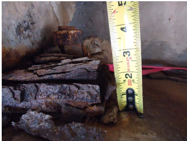
Figure D-54: Corroded, flaky bearing plate
