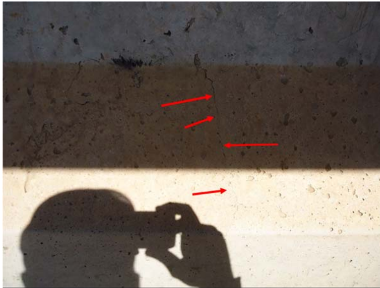
Figure D-57: Crack along the web of girder (5E-S)
