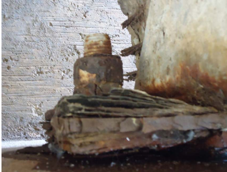
Figure D-33: Corroded and flaky bearing plate (1W-S)
