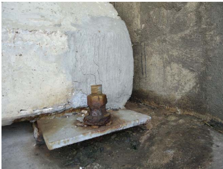
Figure D-7: Repaired concrete on girder end and corroded bolt (1S-W)
