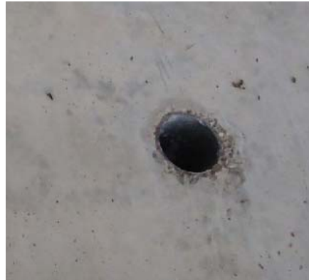
Figure D-16: Spalling around pipe interface with exterior of concrete girder (3E-N)
