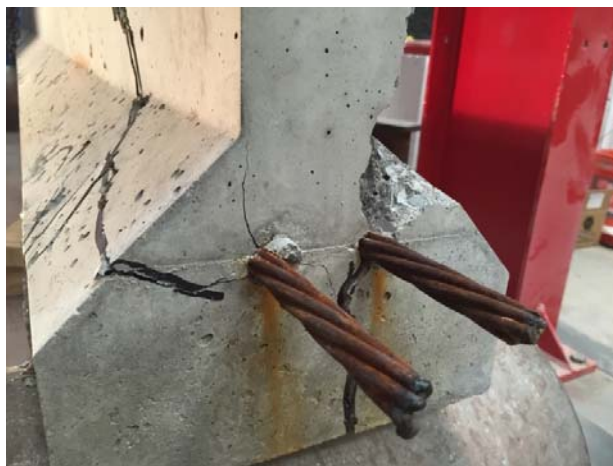
Figure 8-50: Cracking near the prestressing strands at the end of specimen A2N
