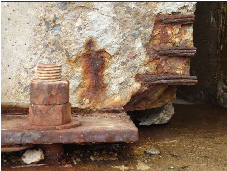
Figure D-32: Exposed prestressing strands of an exposed, exterior girder (1W-N)
