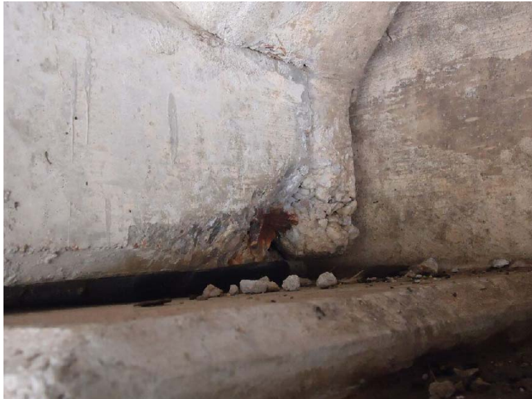
Figure D-66: Exposed rebar, back corner spalled (2S-W)
