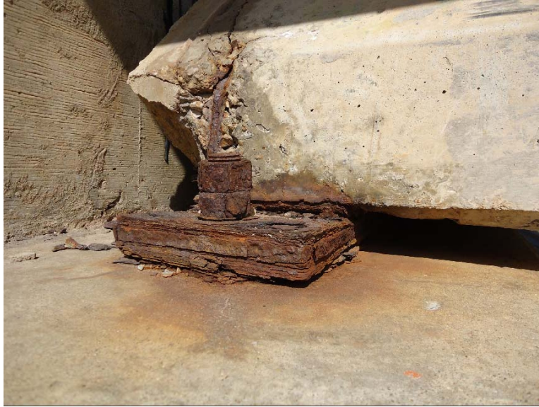
Figure D-59: Corroded bearing plate, exposed rebar, and spalled back corner of girder (5W-S)
