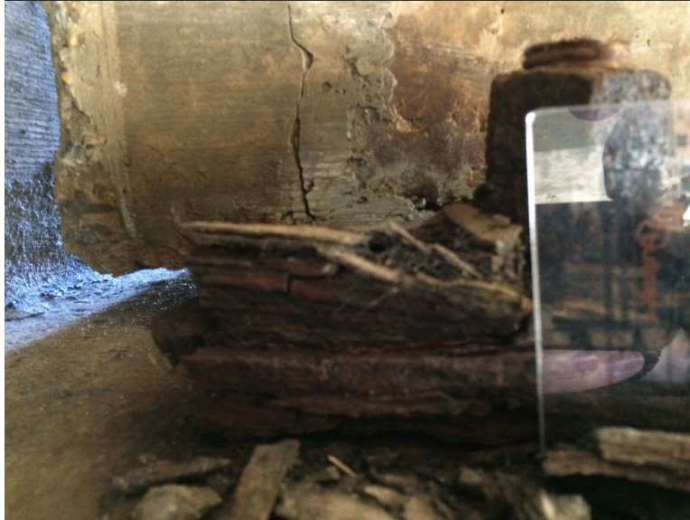
Figure D-55: Vertical crack along interface of girder end and diaphragm (1W-S)
