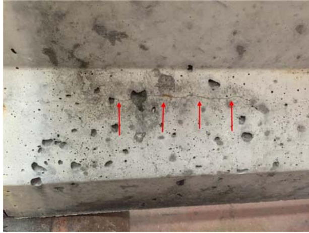
Figure 8-26: Horizontal crack below the web/flange interface of specimen C2NC before testing
