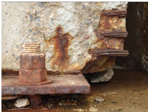
Figure 9-12: Example of exposed prestressing strands
