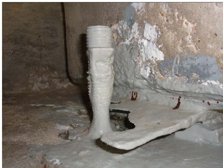
Figure D-62: Severely corroded anchor bolt and bearing plate covered with protective coating (1S-E)
