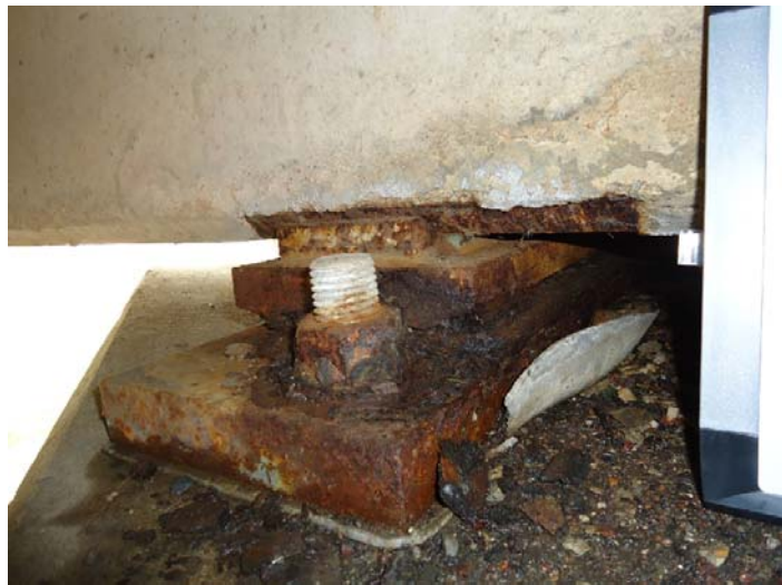
Figure D-20: Corroded bearing plate and minor spalling above the bearing plate (1E-S)
