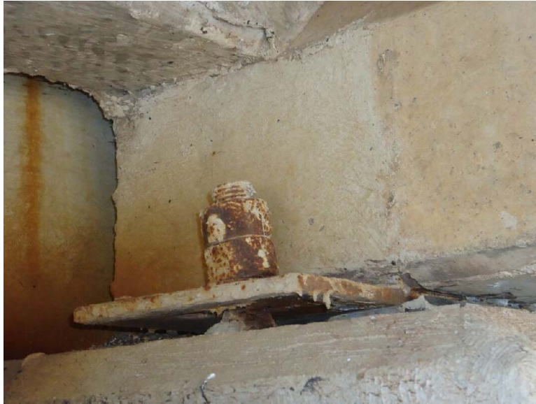
Figure D-39: Corroded anchor bolt (4S-E)
