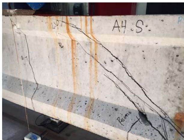
Figure 8-5: Visual map of cracking for shear test of specimen A4SC
