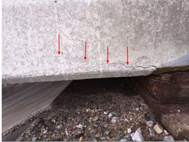
Figure 9-10: Example of crack from damage around the bearing plate
