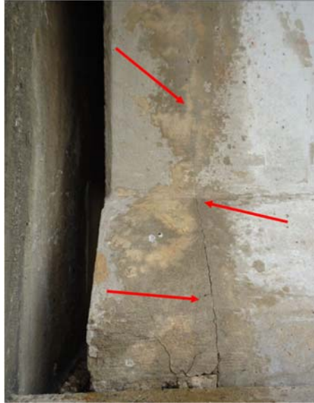
Figure 9-14: Example of vertical cracking along diaphragm and girder
