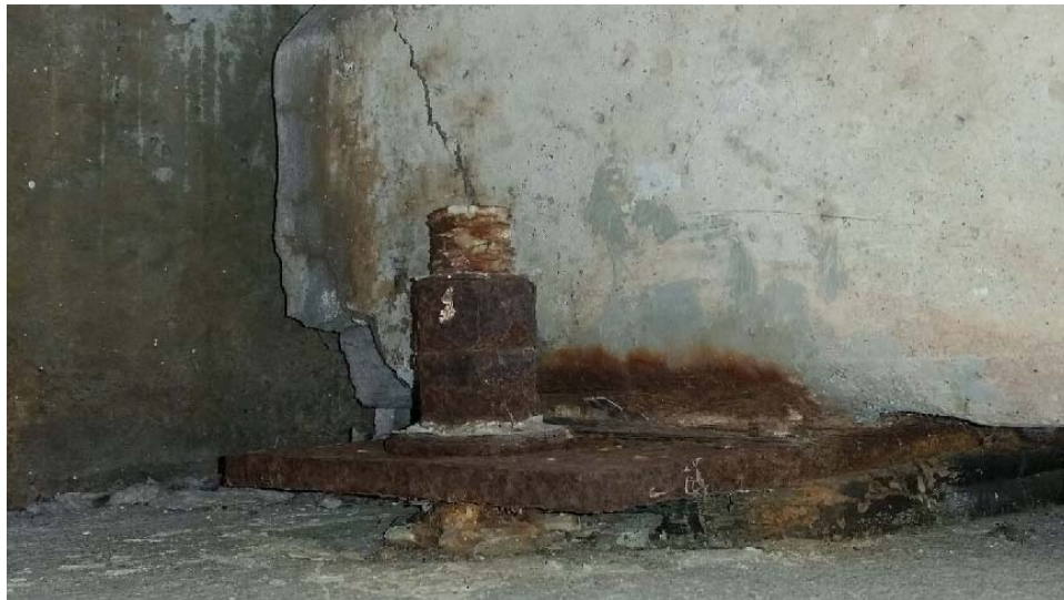
Figure D-36: Back corner diagonal cracking on beam end (11W-S)
