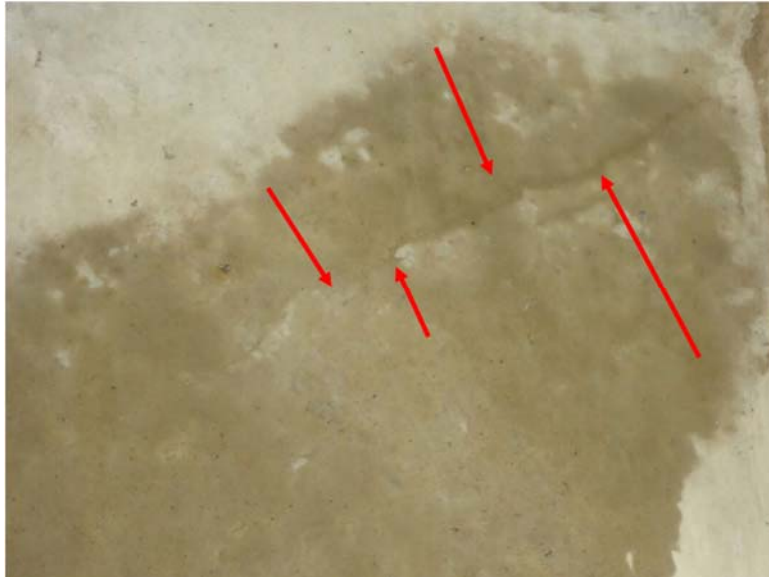
Figure D-67: Diagonal crack from top flange and web interface
