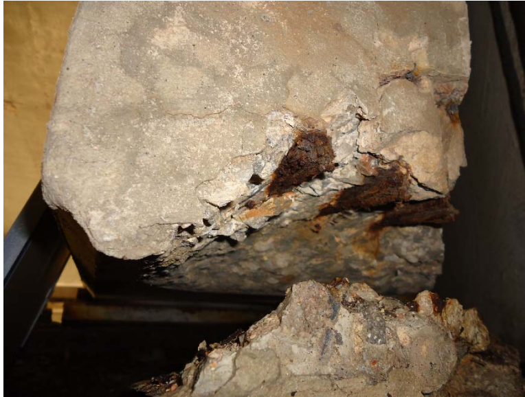
Figure D-22: Spalled back corner and exposed prestressing strands
