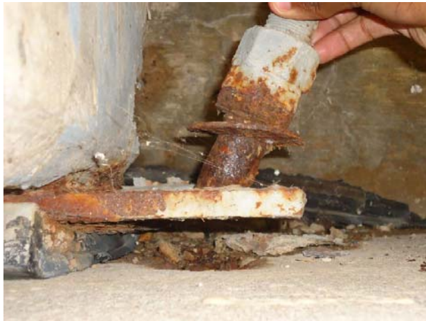
Figure 9-7: Example of corroded anchor bolt
