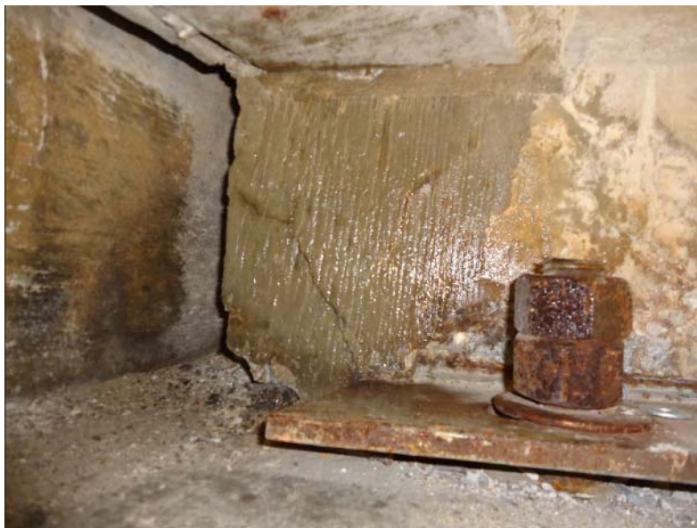
Figure D-19: Back corner diagonal cracking of beam end (5W-S)
