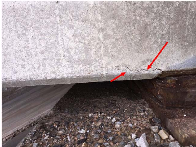
Figure D-26: Cracking from corroded bearing plate into bottom flange (10S-W)
