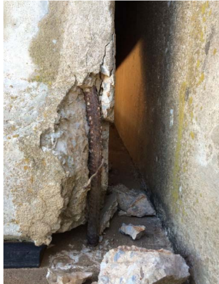
Figure D-49: Exposed vertical rebar due to spalling at the end of exposed, exterior girder (1W-N)
