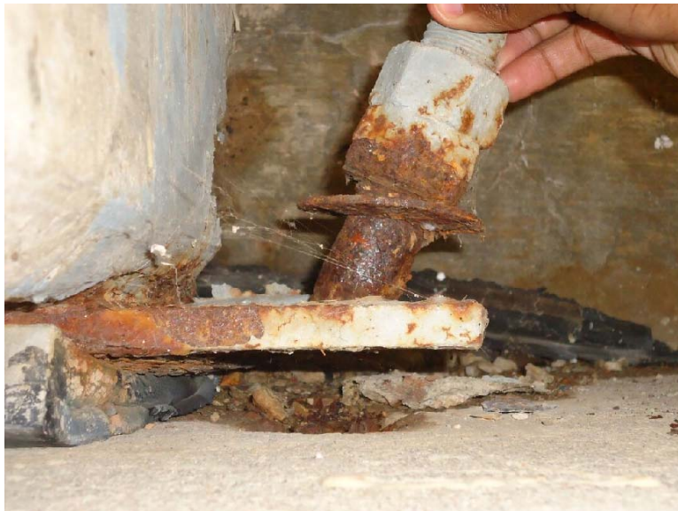
Figure D-34: Corroded anchor bolt that has been sheared in two (7E-S)
