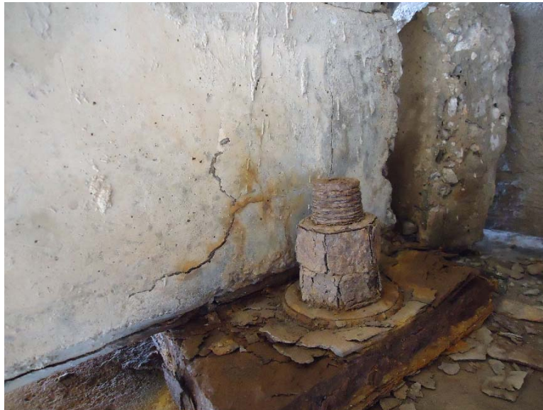
Figure D-48: Corroded bearing plate and anchor bolt, with spalling and cracking above the corroded bearing plate (5W-N)
