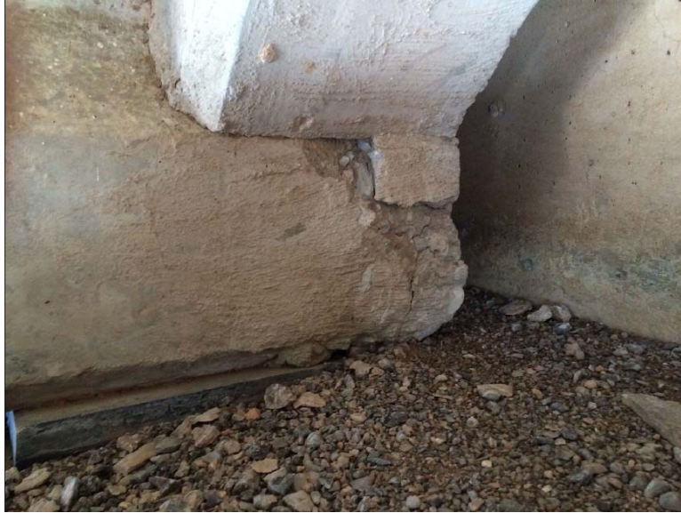
Figure D-51: Spalling at diaphragm and girder interface (3W-N)
