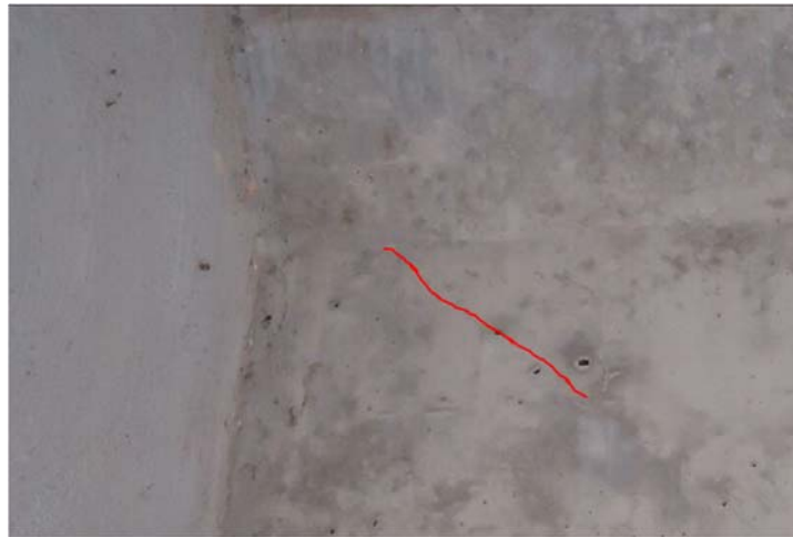
Figure 9-16: Example of diagonal cracking from the top flange and web interface
