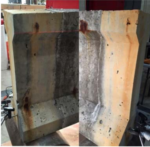
Figure 8-42: Condition of specimen A2SC prior to testing
