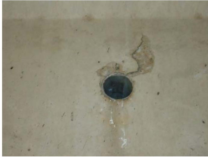
Figure D-37: Spalling and cracking above pipe in web (1N-E)
