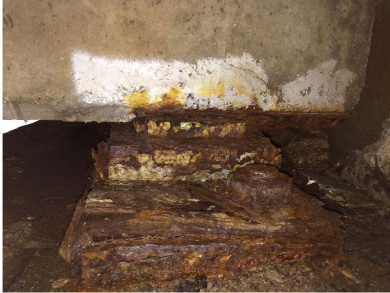
Figure D-25: Corroded, and deteriorated bearing plate (8N-E)
