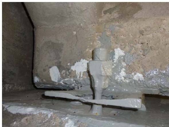
Figure 9-8: Example of coated, damaged anchor bolt and nut
