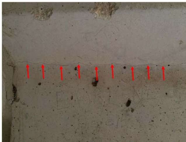
Figure 9-15: Example of horizontal cracking along the top flange and web interface
