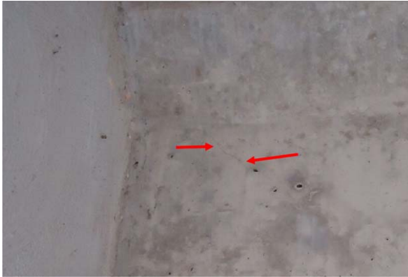
Figure D-8: Diagonal cracking on the web of the beam (3N-W)
