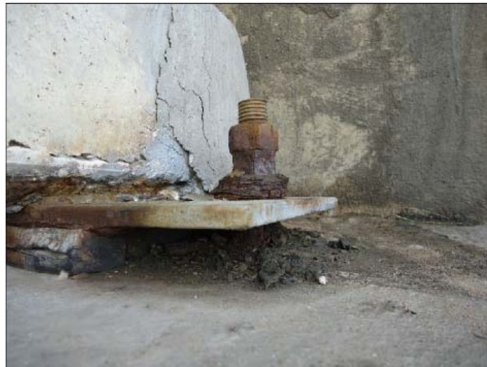
Figure D-5: Corroded anchor bolt (1S-W)
