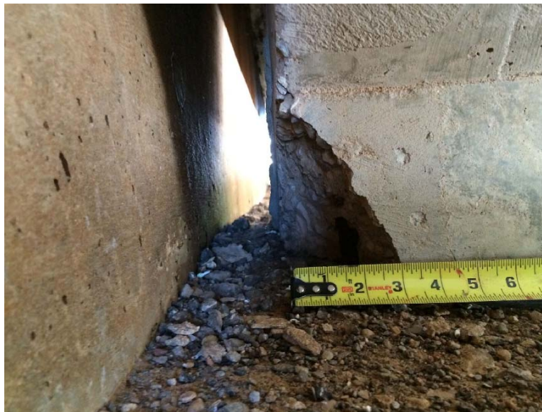
Figure D-50: Spalling resulting from back corner diagonal crack (2E-N)
