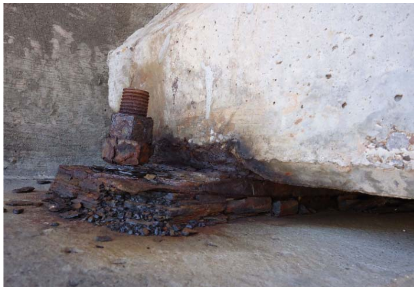
Figure D-52: Corroded bearing plate, bolt, and nut along with spalling above the support of an exposed, exterior girder (1E-N)
