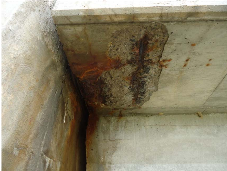
Figure D-6: Exposed rebar, showing insufficient concrete cover at end of bridge deck (1N-W)
