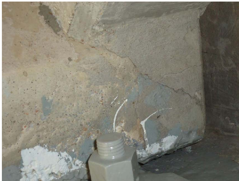
Figure D-64: Diagonal crack at back corner of girder end (2S-W)
