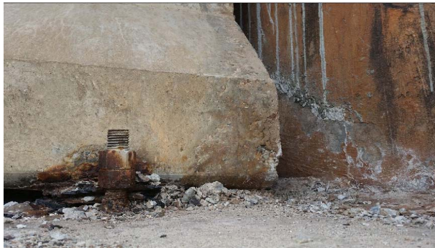
Figure D-30: Corroded anchor bolt and spalling along bottom of girder and girder end (5N-E)
