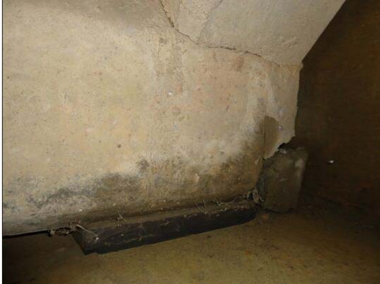
Figure D-10: Back diagonal crack in the beam end (3N-E)
