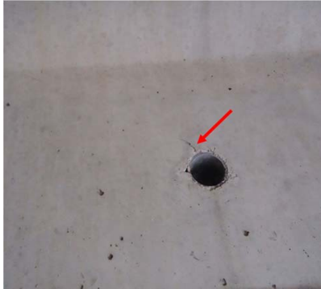
Figure D-14: Crack from interior pipe that runs through web of beam (4E-N)
