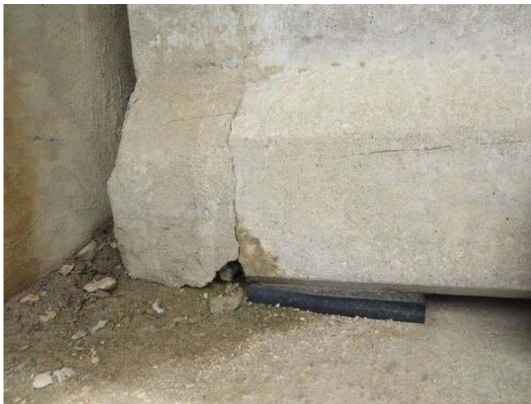
Figure D-11: Separation at the diaphragm and girder end (1N-W)
