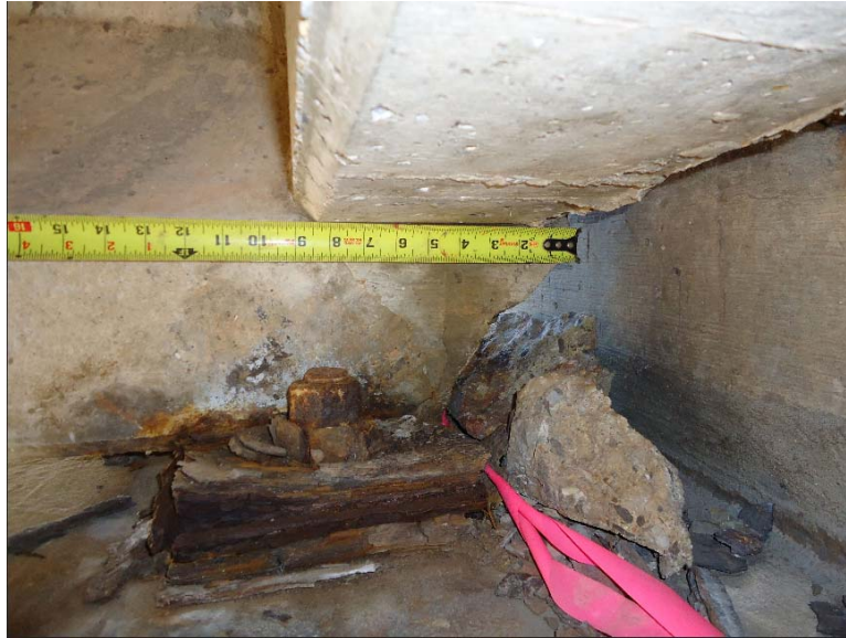
Figure D-53: Corroded bearing plate and spalling from a diagonal back corner crack with a maximum width of approximately four inches
