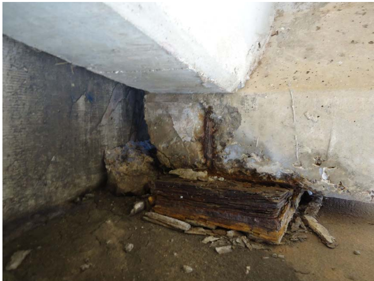
Figure D-56: Exposed rebar, corroded, flaky bearing plate, and spalling of concrete (5E-N)
