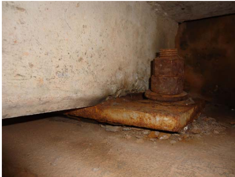
Figure D-44: Corroded bearing plate and anchor bolt with spalling above the support (5E-S)
