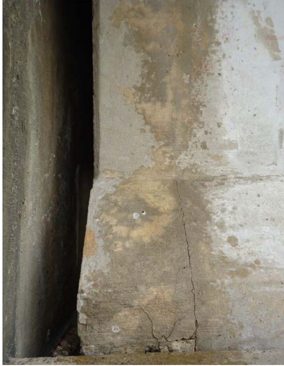
Figure D-65: Vertical crack at girder/diaphragm interface (1N-W)
