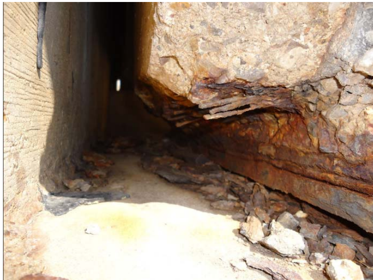
Figure D-58: Diagonal back corner spalling and exposed prestressing strands (5W-S)
