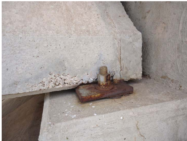
Figure D-46: Spalling above the corroded bearing plate (1W-N)
