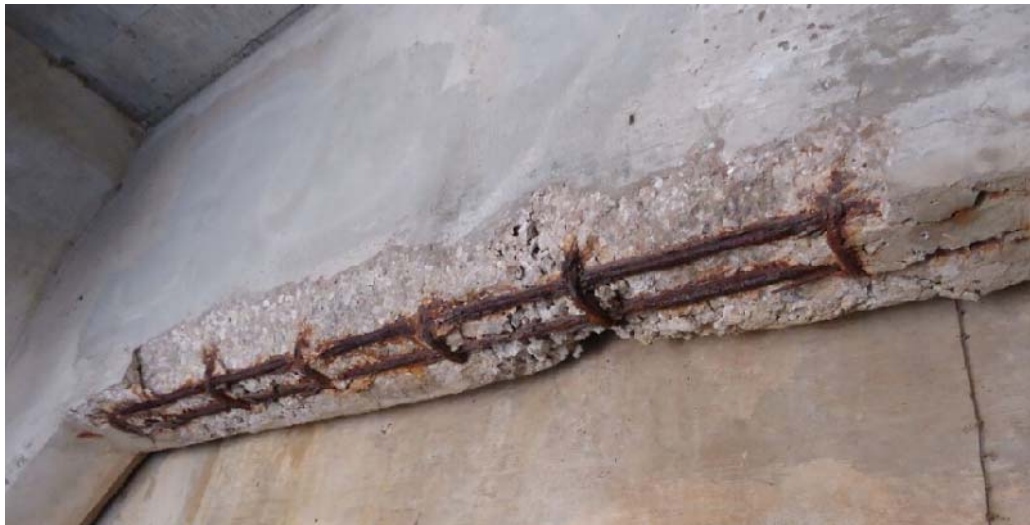
Figure D-68: Corrosion on underside of end diaphragm with exposed and corroded rebar
