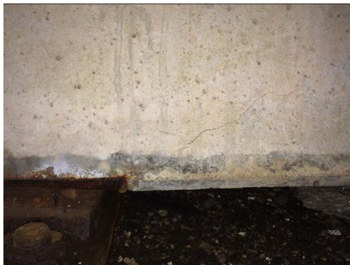
Figure D-21: Diagonal crack in bottom flange of beam from corroding support (10W-N)
