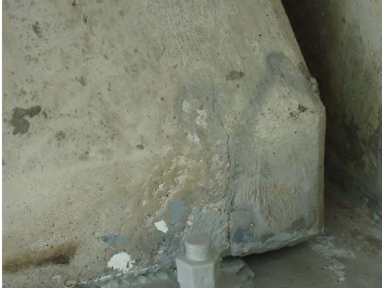
Figure D-63: Vertical crack at girder and diaphragm intersection (1S-W)
