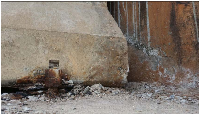
Figure 9-9: Example of spalling above bearing support
