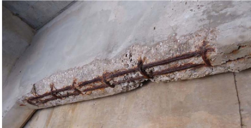
Figure 9-17: Example of diaphragm deterioration
