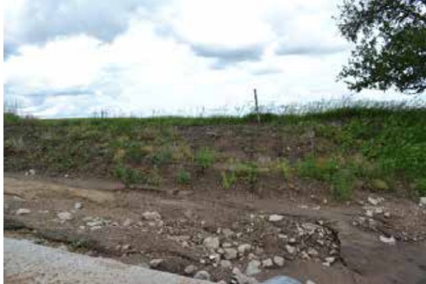
Figure 5.27: Sediment Deposited on Top of Rock Riprap on Downstream Side of Structure
