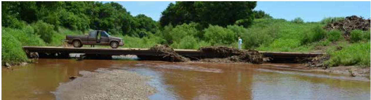
Figure 2.2: Woody Debris Trapped on Upstream Side of Low-Water Bridge in Sumner County, Kansas
