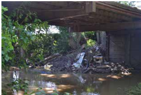
Figure 5.40: Right Abutment with Original Wood Planks
