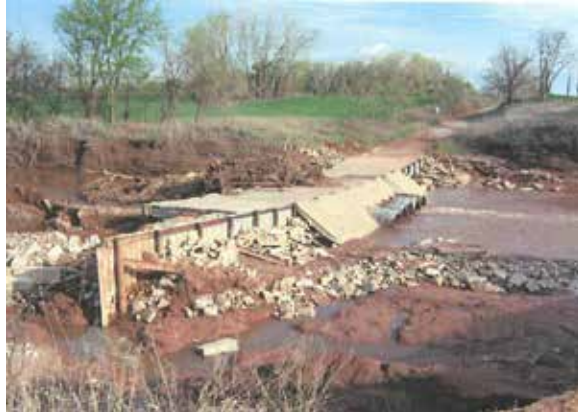
Figure 5.71: Downstream Side of Old Structure with Washed-Out South Approach
