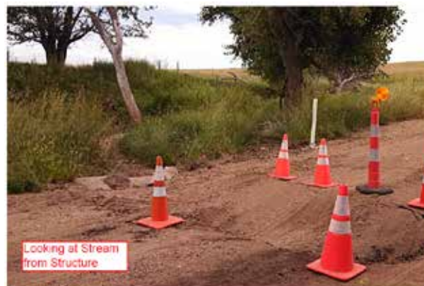
Figure 5.26: Partially Collapsed Culvert Deck
