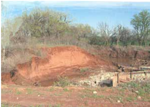
Figure 5.72: Washed-Out South Approach to Old Structure
