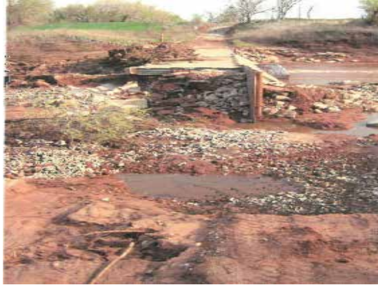
Figure 5.73: Old Structure Viewed from Washed-Out Approach
