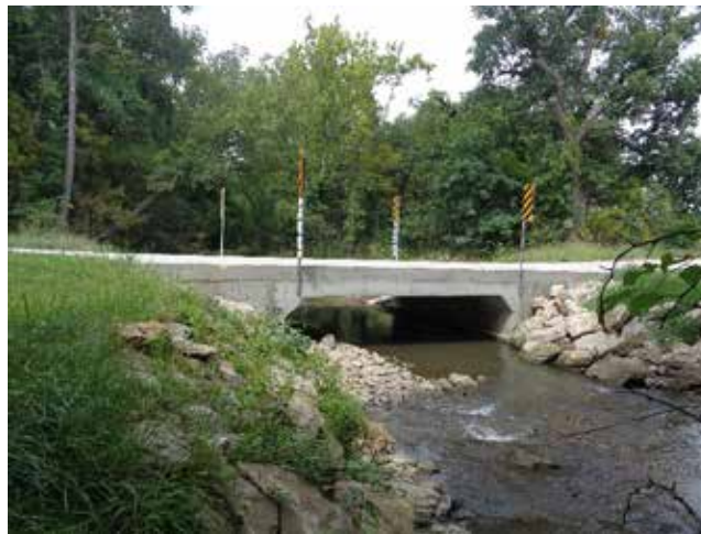
Figure 1.5: Low-Profile Bottomless Culvert in Johnson County, Kansas
