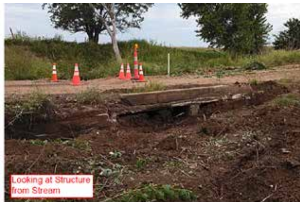
Figure 5.25: Old Structure Filled with Sediment
