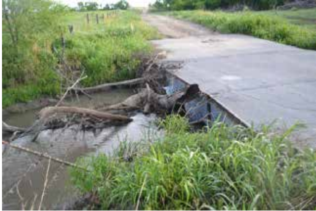
Figure 5.33: Timber Build-Up on the Upstream Face of Structure
