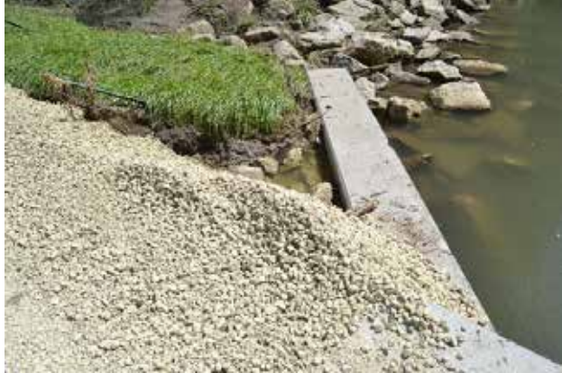
Figure 5.79: Scouring Behind the Upstream Right-Bank Wing Wall
