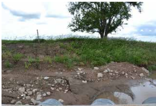
Figure 5.23: Washed-Away Aggregate Stabilization on Downstream Left Bank
