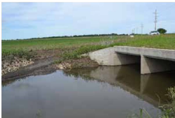
Figure 5.44: Upstream Wingwall with Riprap Stabilization Covered in Silt
