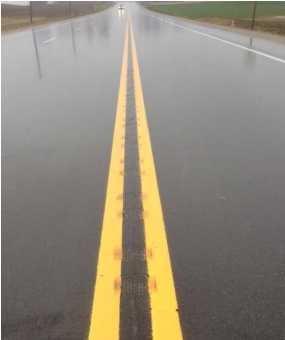
Figure 35 - STH 26 longitudinal joint, photographed 3/31/16
