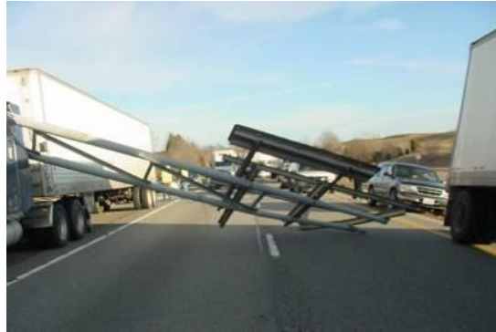
FIGURE 3-2 Example of overhead sign failure (FHWA, 2013)
