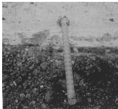
Figure A-9: Deformed Tie Bar
