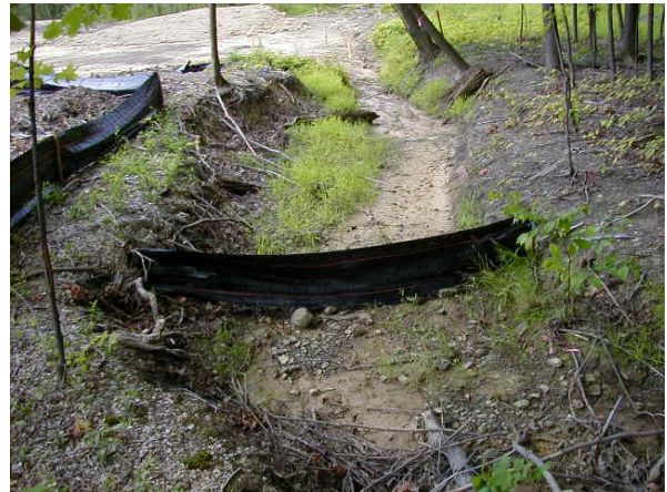
Figure A-27: Improper Use of Silt Fence as a Check Dam
