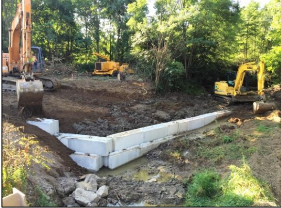
Figure 25 The sill, at right angles with the bank, is visible prior to backfill and placement of buried riprap.
