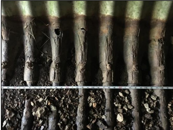
Figure 68 Corrosion 8 feet from the upstream end.
