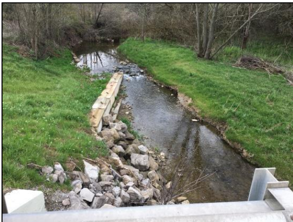
Figure 26 After one winter and spring high flows note the stability on the river right bank and the location of the scour downstream from mid-way along the vane.
