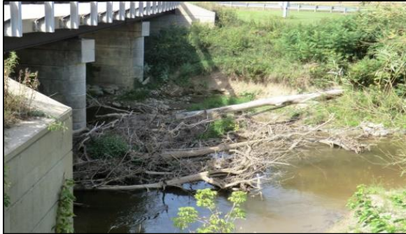
Figure 43 Debris accumulation on the left pier and erosion on the right bank.
