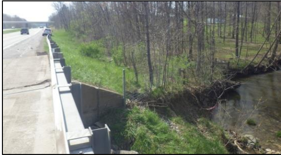
Figure 565 Looking upstream at the eroding roadway embankment.
