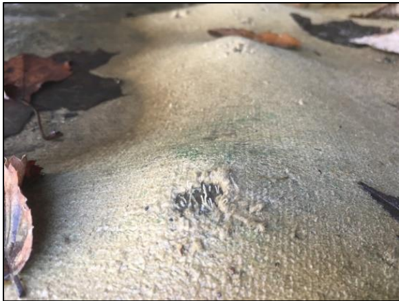
Figure 13 Abrasion over the CMP's bolts.
