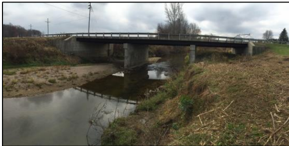
Figure 44 Viewed looking downstream, a low bar on left and a high depositional floodplain bar in the right span.
