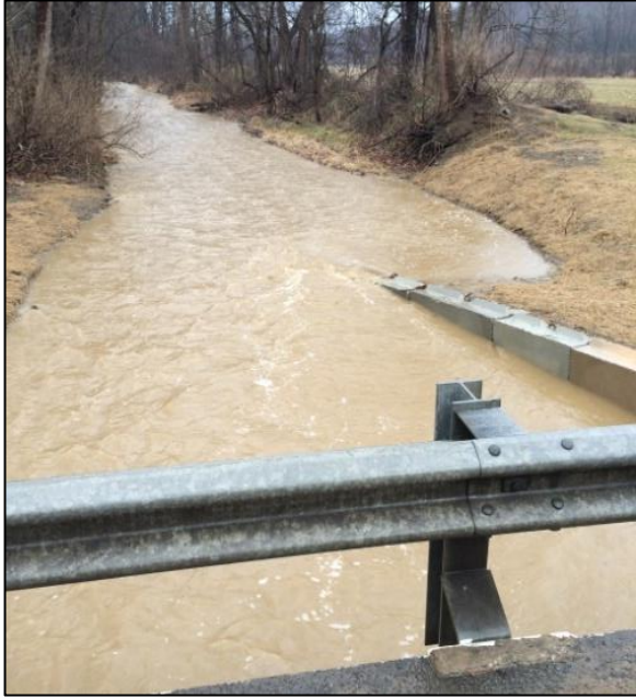
Figure 21 Moderate flow is shifted smoothly to the center of the span without turbulence or eddies.
