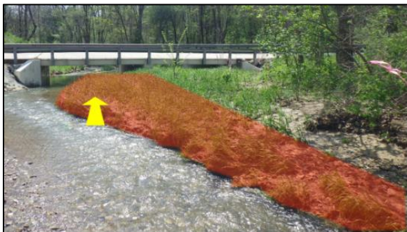
Figure 17 The highlighted portion of the floodplain bar was removed to align low and intermediate flows with one span. The second span provides hydraulic capacity for large events.
