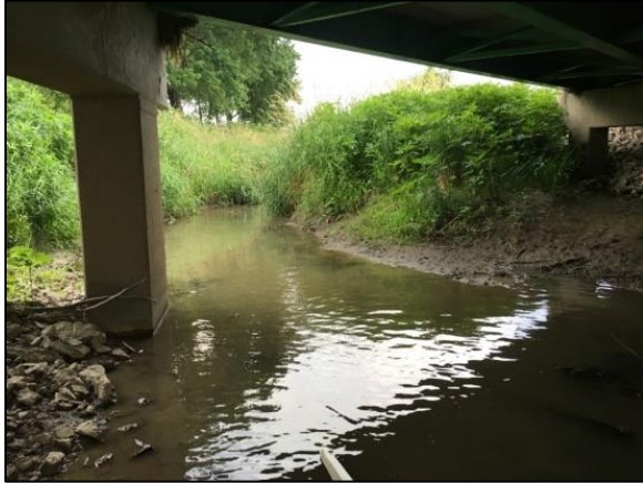
Figure 51 Poorly aligned channel viewed looking upstream.
