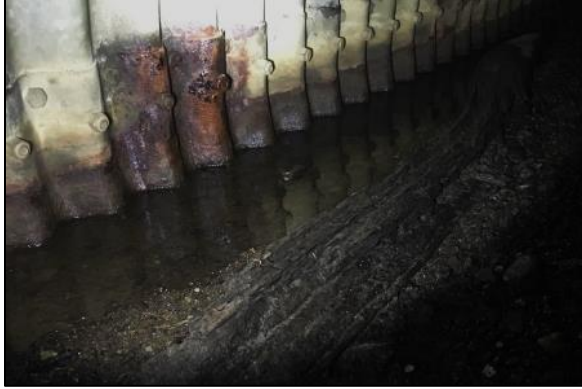
Figure 69 Beyond 50 feet the CMP is less corroded.
