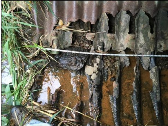
Figure 1. Severe corrosion at the upstream end of the CMP.
