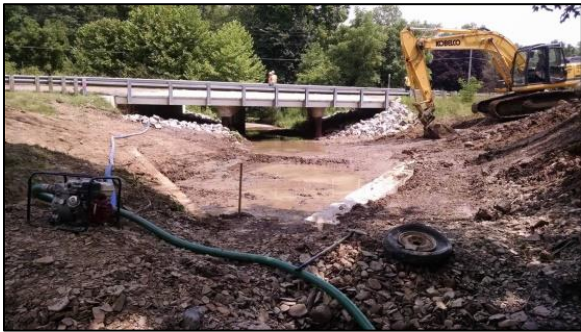
Figure 31 Viewed looking downstream at the cross vane.
