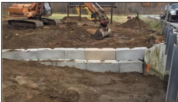
Figure 20 The downstream end of the vane at the bridge abutment.
