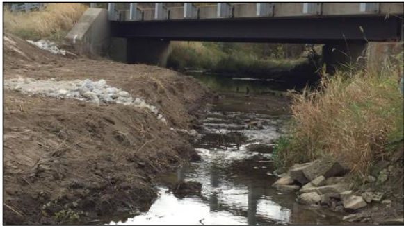
Figure 55 Minimal excavation below the bench stage to align the low and intermediate flows.
