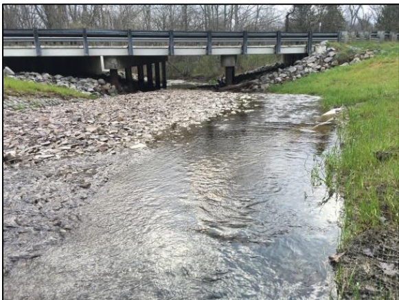
Figure 34 Looking downstream the vane mostly obscured by accumulated bed material. Note the channel width should be similar to the width between the piers.
