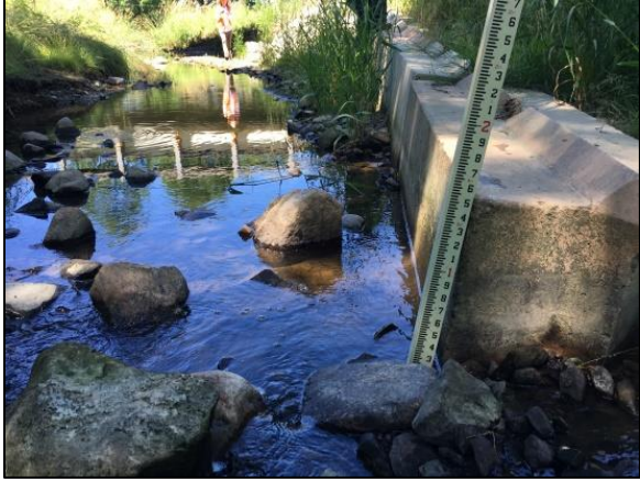
Figure 27 The upstream end of the vane is stable but has become more exposed from the vane inducing scour of a riffle.
