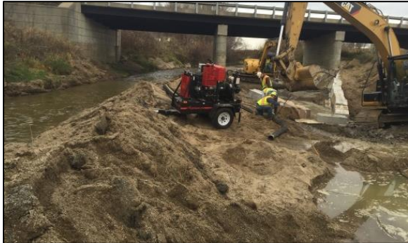
Figure 46 Construction in a sand bed channel by diverting flow and dewatering with a 6 inch pump.
