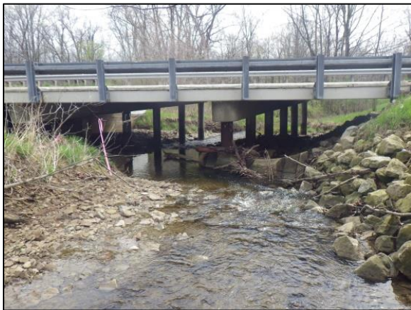
Figure 29 Poor alignment of low and intermediate flows with debris collecting on the right piers.
