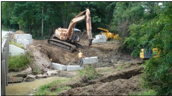
Figure 24 The footer course of block of the vane and the sill being set.
