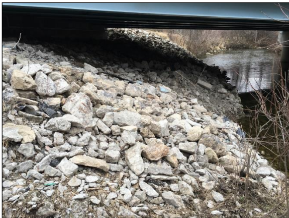
Figure 64 Concrete rubble placed instead of Flexamat.
