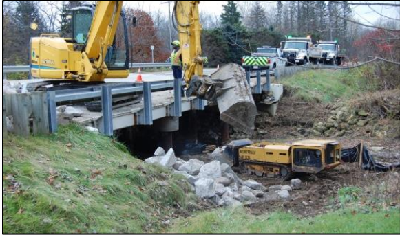
Figure 30 The remote control excavator removed sediment and placed rock under the bridge deck.
